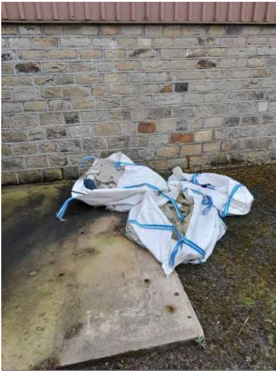
3: Looking south, towards the bagged suspected asbestos sheeting.
