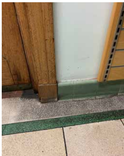
4.8.16 - Architrave to Boys WC (Rm.23)
