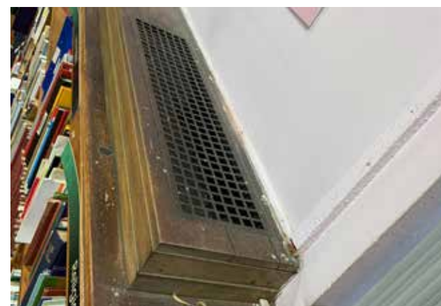
4.6.11 - Ventilation in Local History Library (Rm.68)
