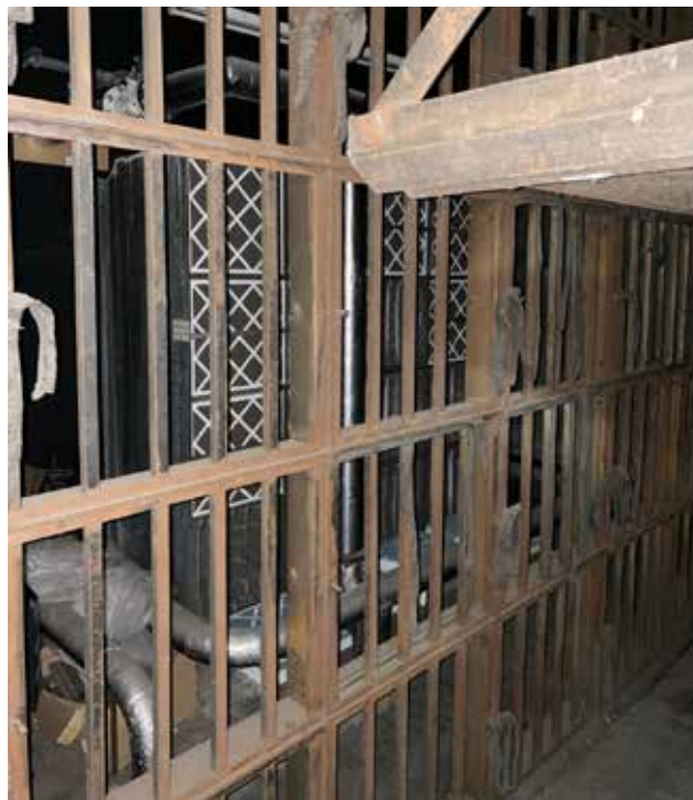
4.8.12 - Air Filter Chamber (Rm.37)
