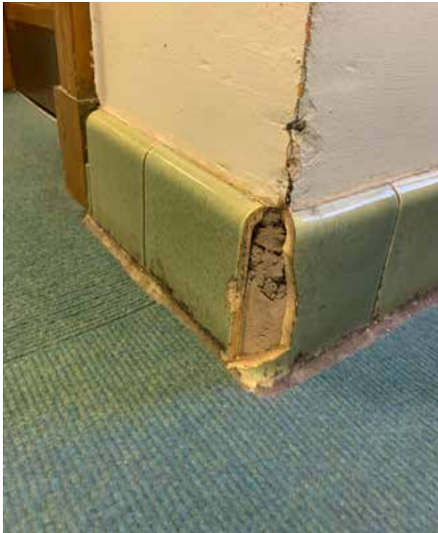
4.6.5 - Skirting to First Floor Stair Lobby (Rm.71)
