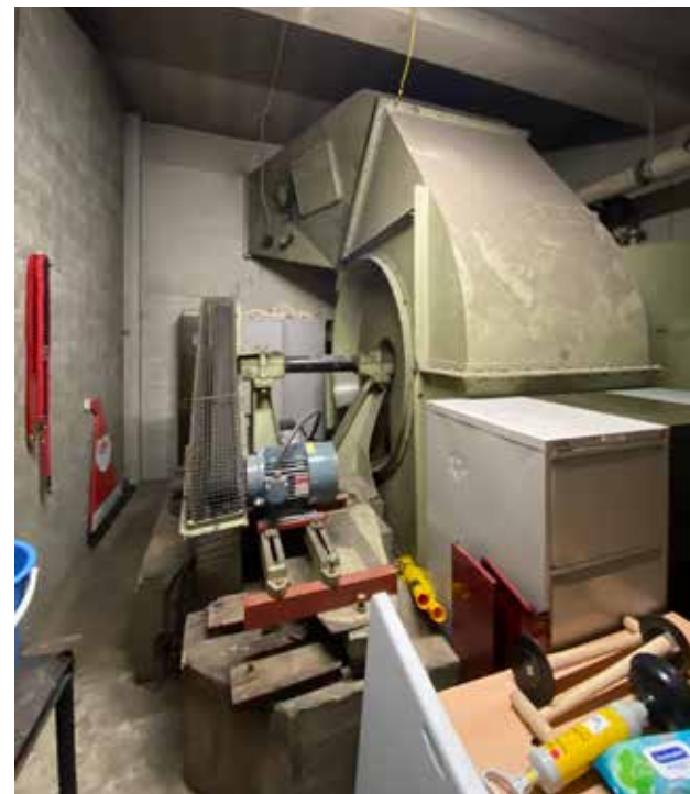
4.8.13 - Plant Room (Rm.38)
