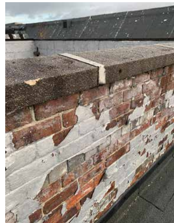
4.4.17 - Deteriorating roof parapet
