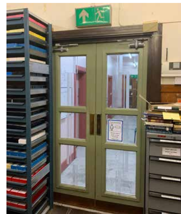
4.6.15 - Doors in Reference Archive (Rm.66)
