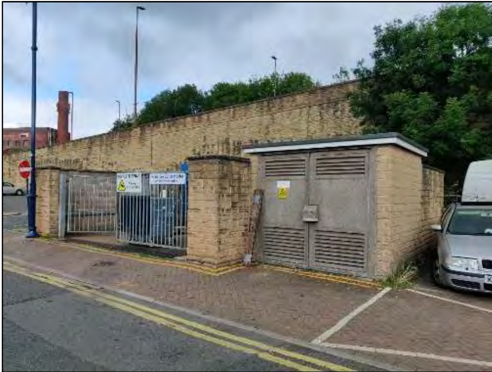
Photo K: View of the bin storage area and electrical substation next to the car park, facing north.
