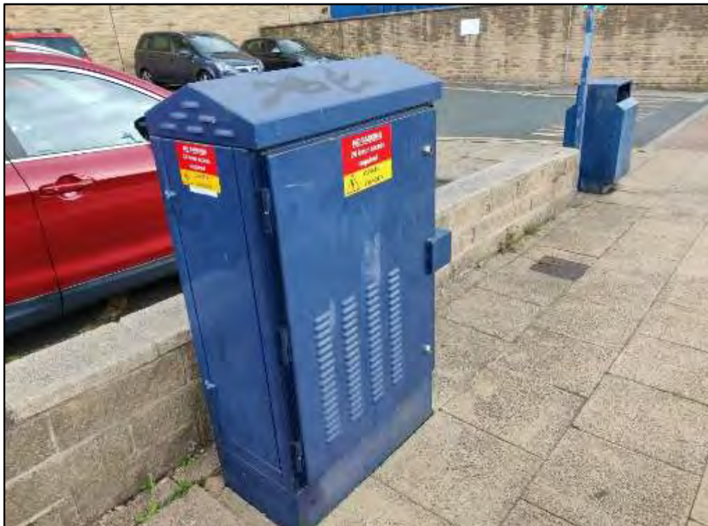
Photo L: View of the electric fuse box next to the carpark, facing east.
