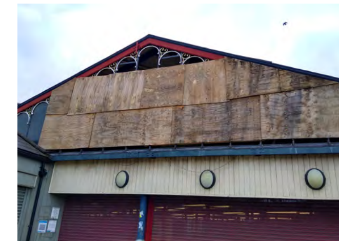
Figure 7.1.5 Vandalism and damage to glazing is common
