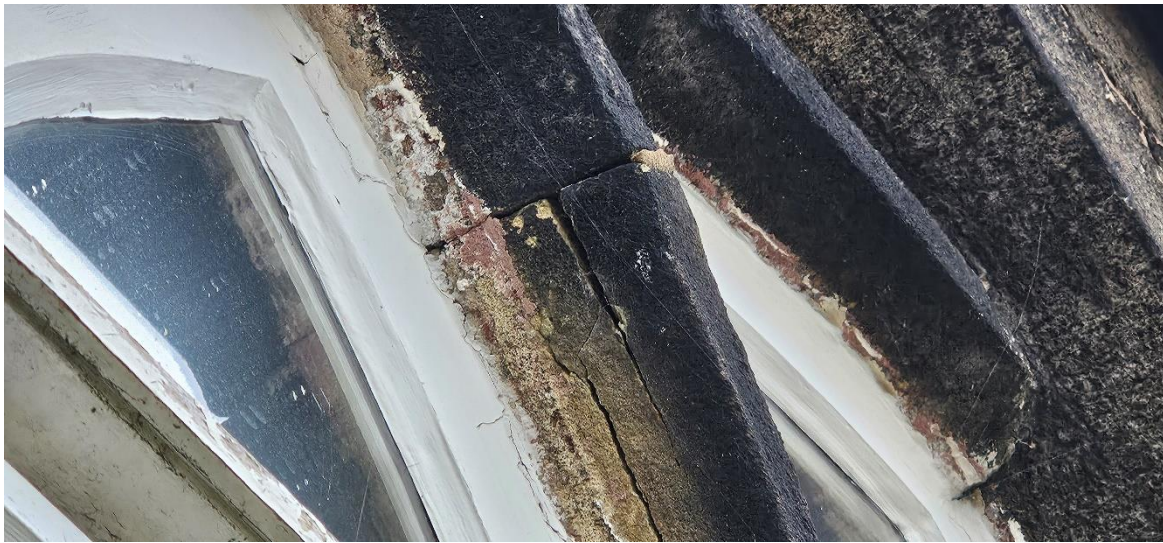
Photo 7: Stonework deterioration with splits and cracks in sections of stone arches.
