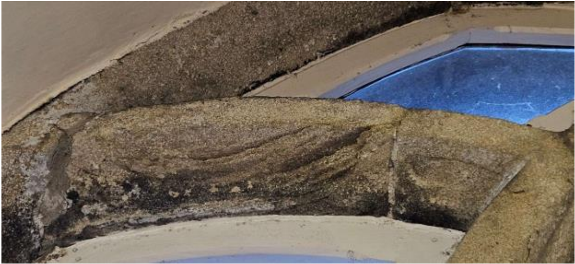
Photo 19: Worn and previously pointed sections evident to stonework internally.
