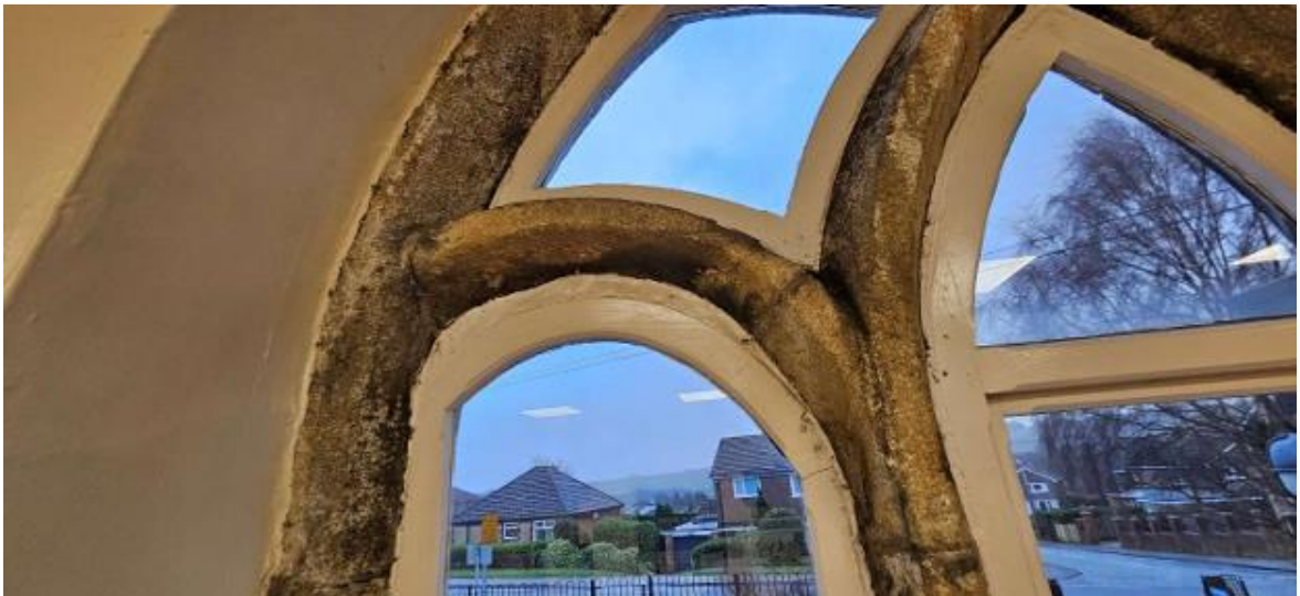
Photo 20: Excessive gaps between timber frames and stonework to previous installation evident.
