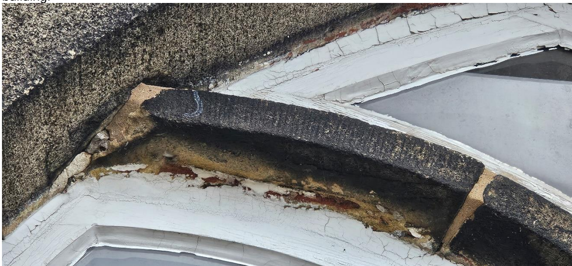
Photo 9: Example of previous pointing repairs to fill gaps between sections of stone arch.
