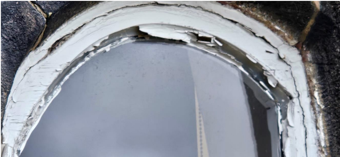
Photo 12: Gaps opening up between top of window frame and seal also evident is missing sections of glazing putty exposing edge of glazing pane.
