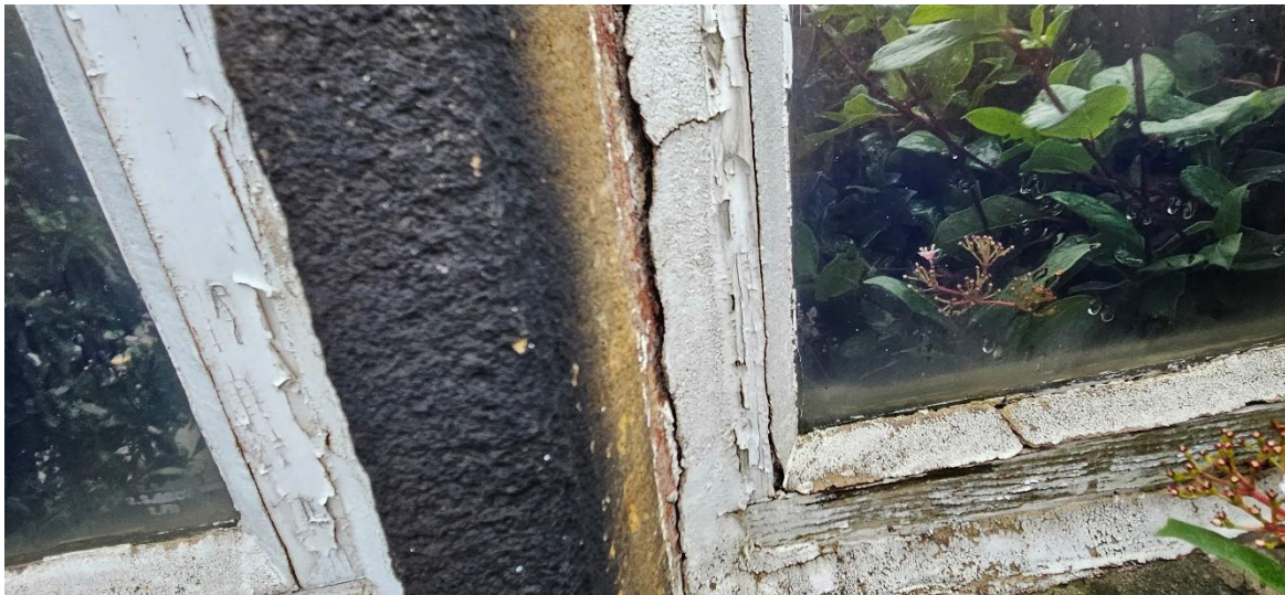
Photo 8: Putty infill and mortar repairs are cracked and lifting allowing moisture to penetrate into building.
