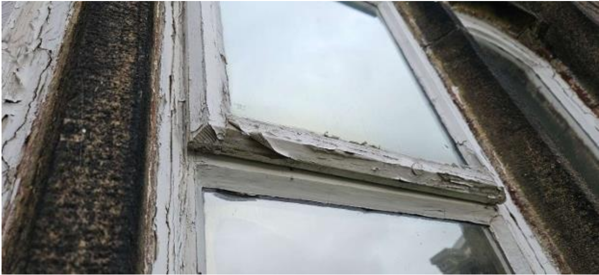
Photo 10: Window opener with gaps where frame has twisted / warped.
