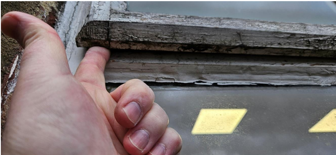
Photo 11: Extent of gap between frame and opener demonstrated with finger used for scale reference point.
