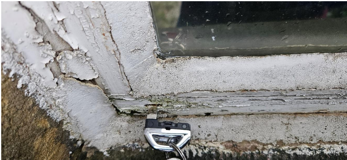
Photo 5: Rotten timber window frames with car key easily pushed into soft and saturated timber.
