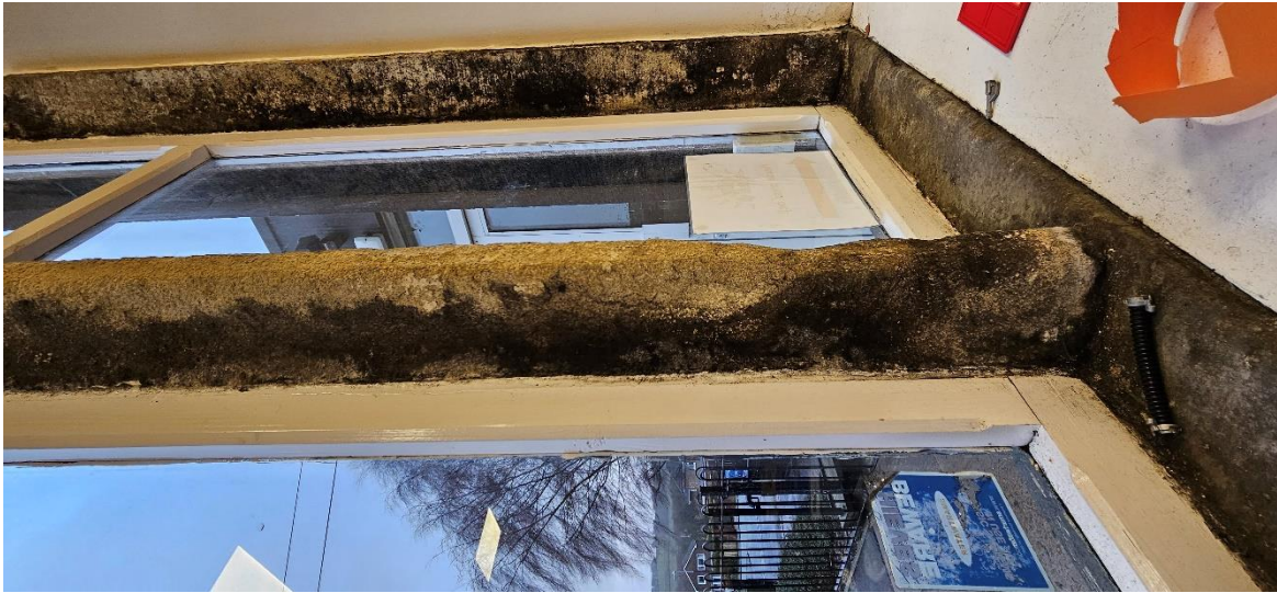
Photo 16: Further example of wear and staining to internal stonework from penetrative damp and condensation.
