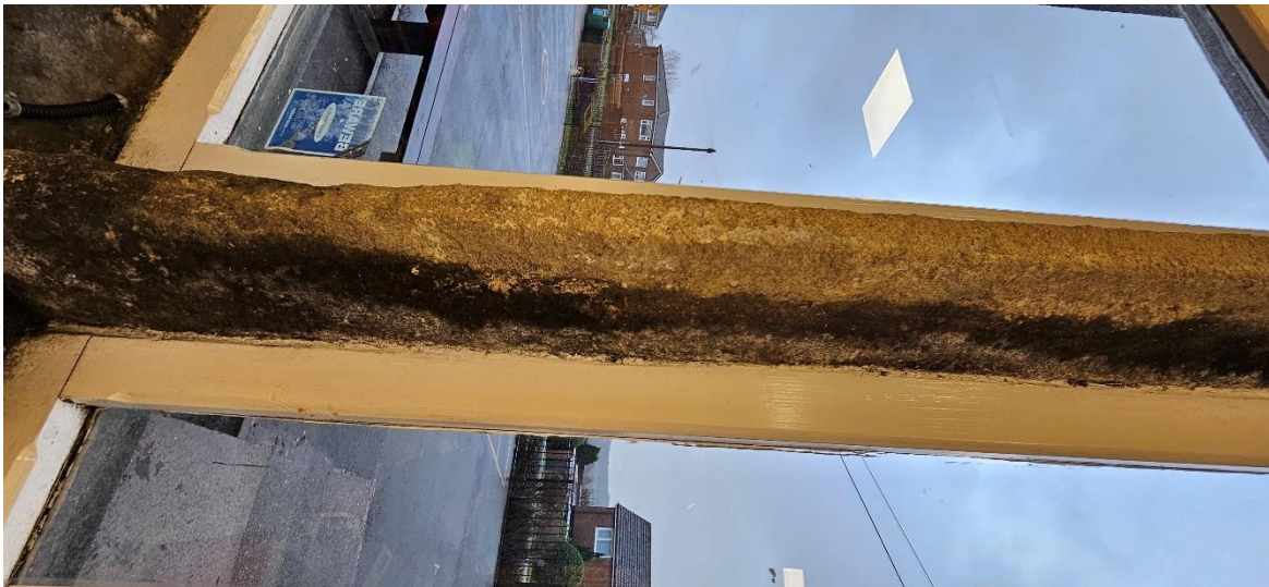
Photo 17: Further example of worn stonework.
