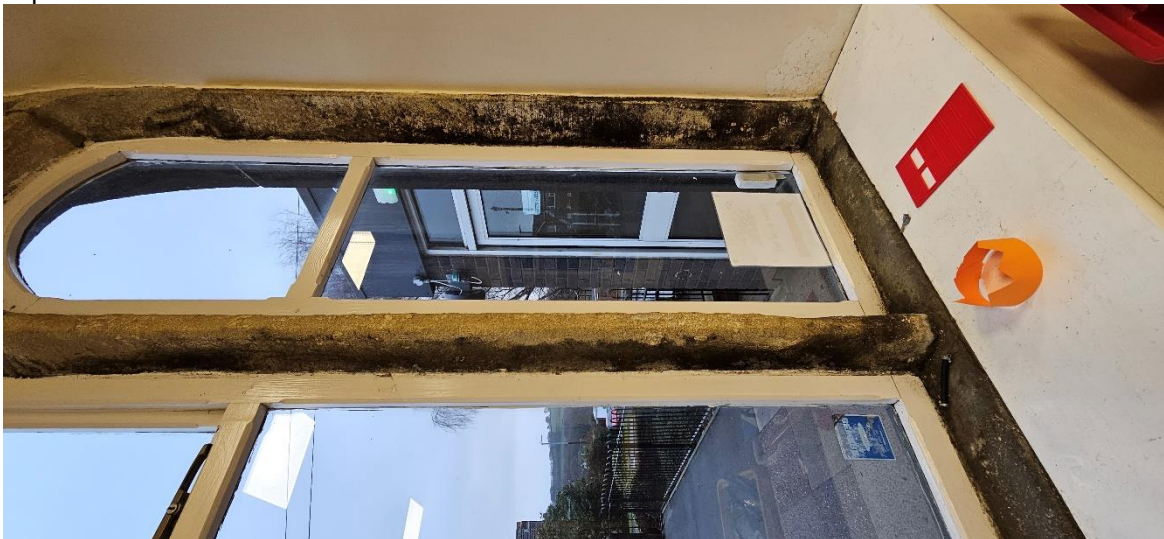
Photo 14: Internal view of window showing black mould, moisture staining and wear to stonework.
