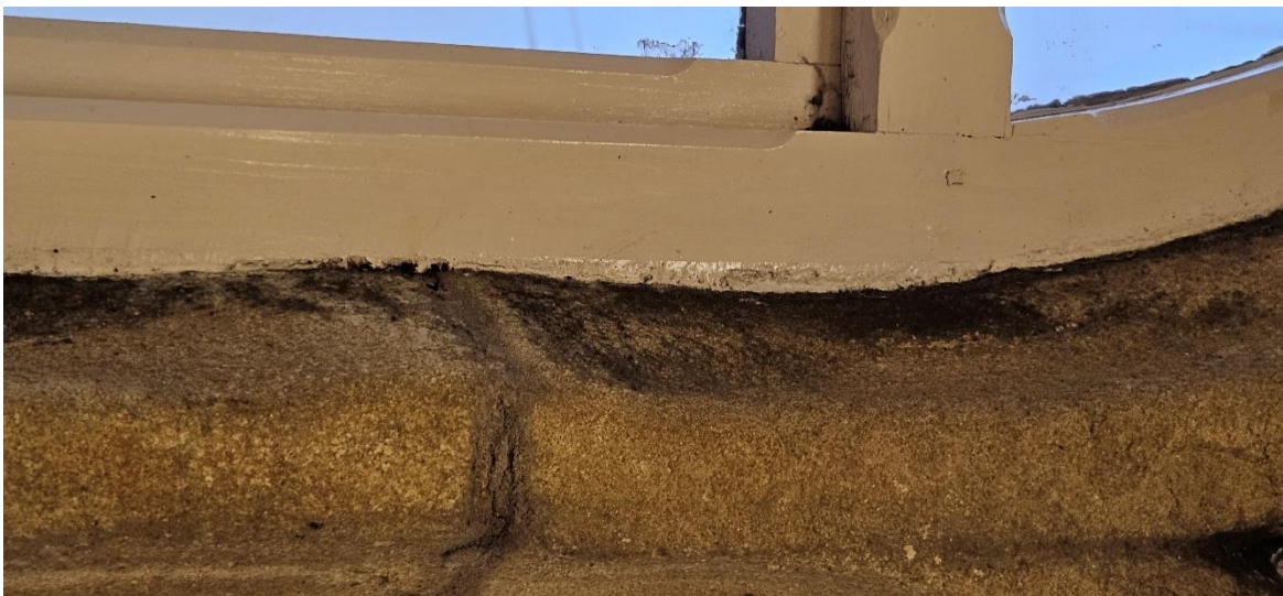
Photo 18: Further example of uneven edges to stonework and how gaps between the timber frame and stonework have been filled.
