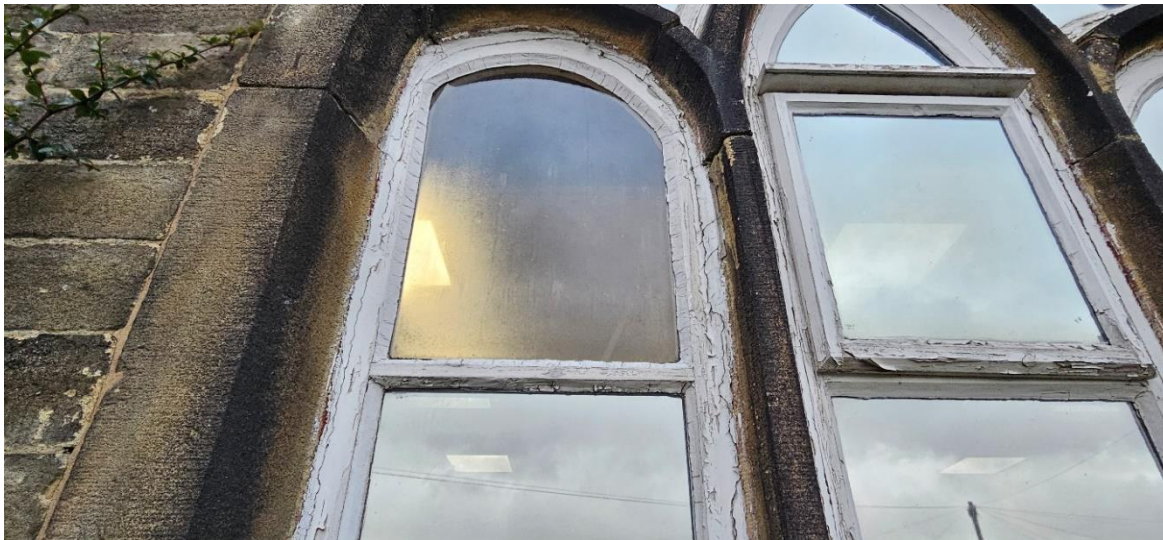
Photo 4: General view showing poor condition of timber framed windows inset in between stone arches.
