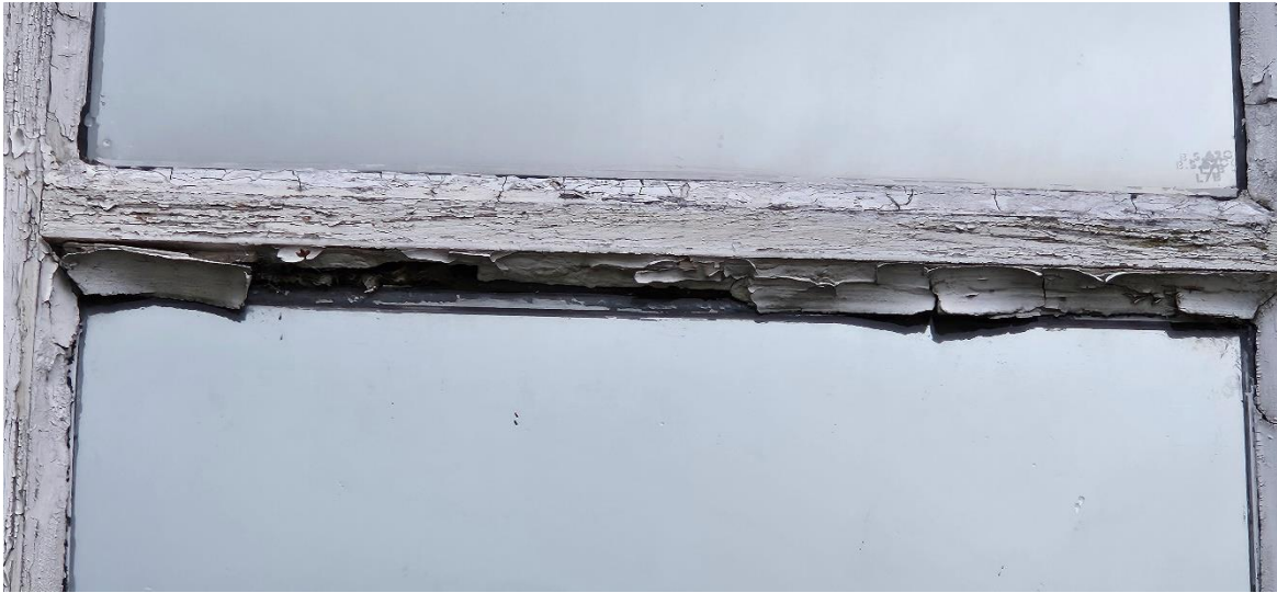
Photo 13: Worn and deteriorated timber glazing bead and missing glazing putty which holds glass in place.
