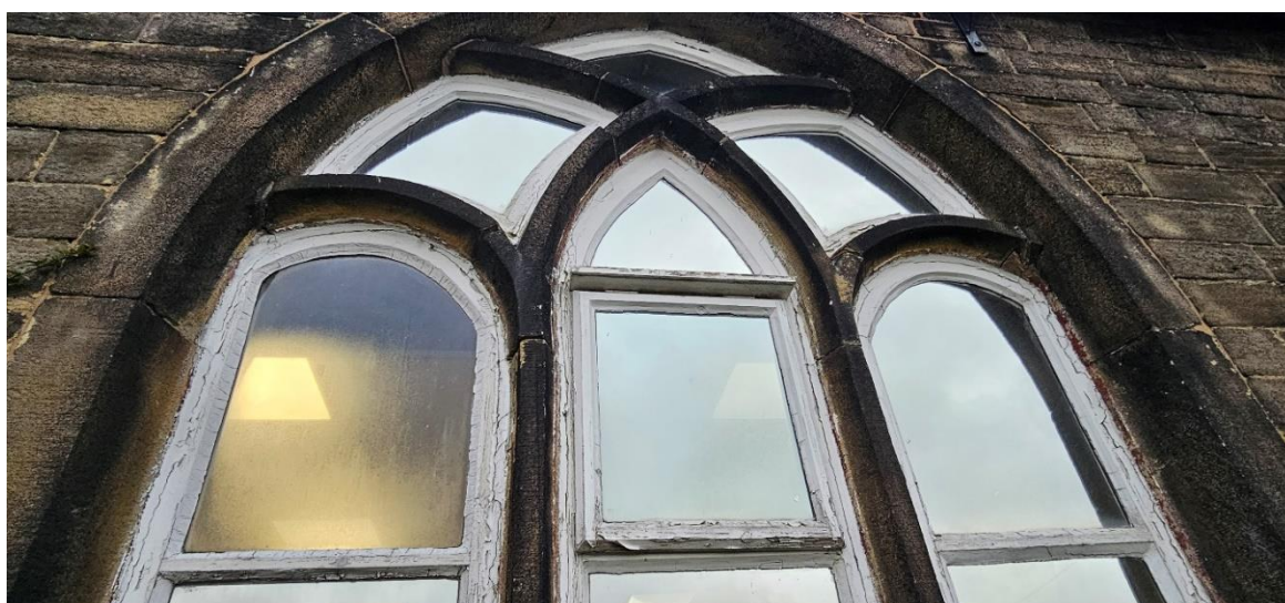
Photo 2: Typical detail of arched window, showing stonework and rotten timber framed single glazed windows.
