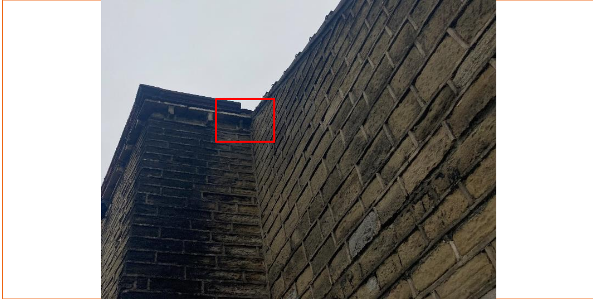
Figure 5 Showing the crevice where the extension meets the main building (PRF 5)
