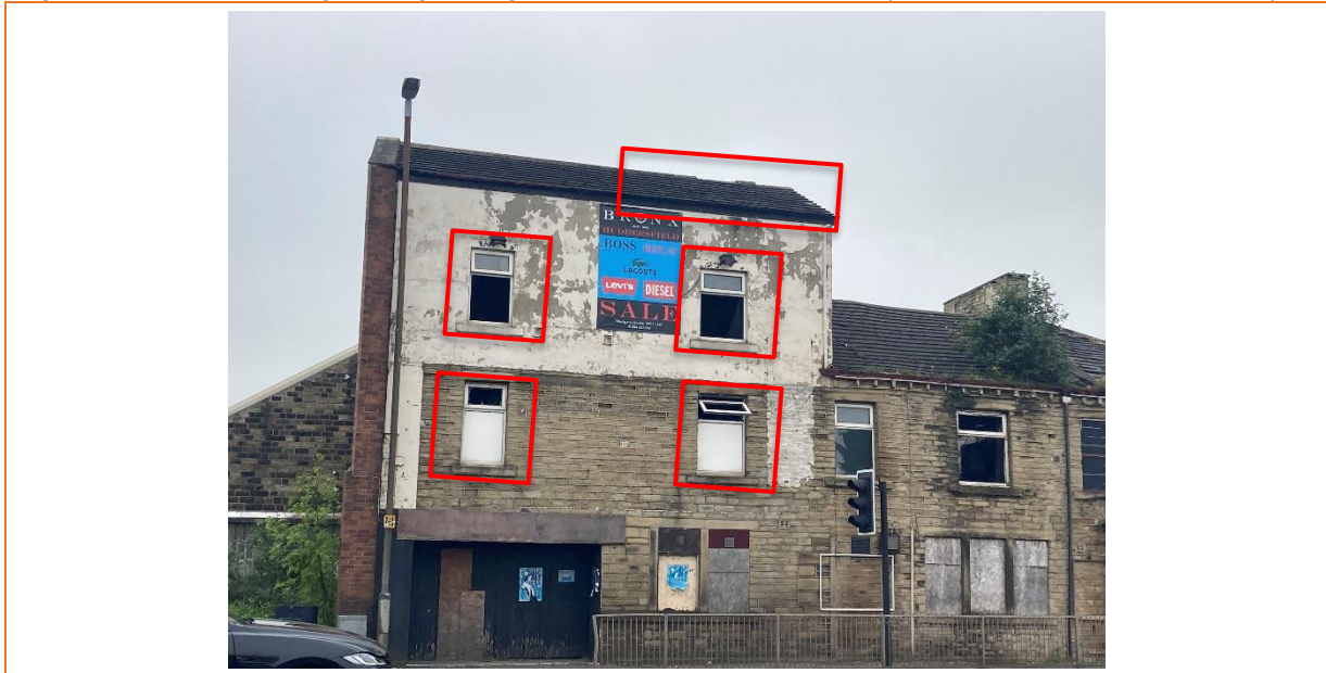
Figure 18 Showing damaged ridge tiles and broken windows (PRF18, AP7, AP8, AP9, AP10)
