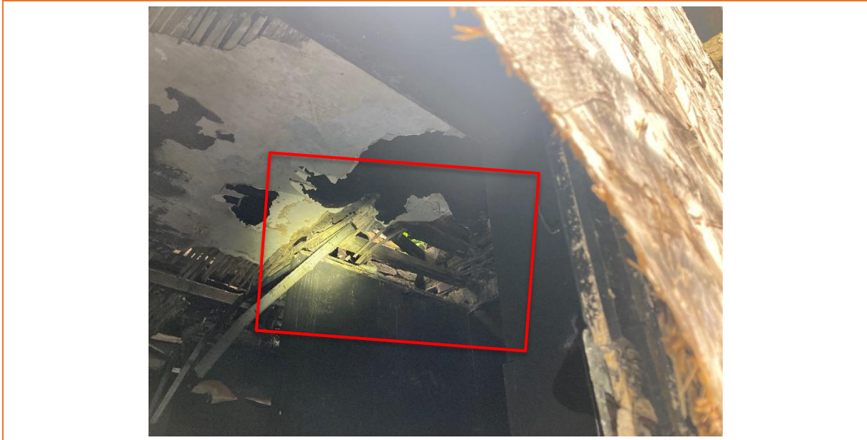
Figure 20 Showing damaged roof (AP11)
