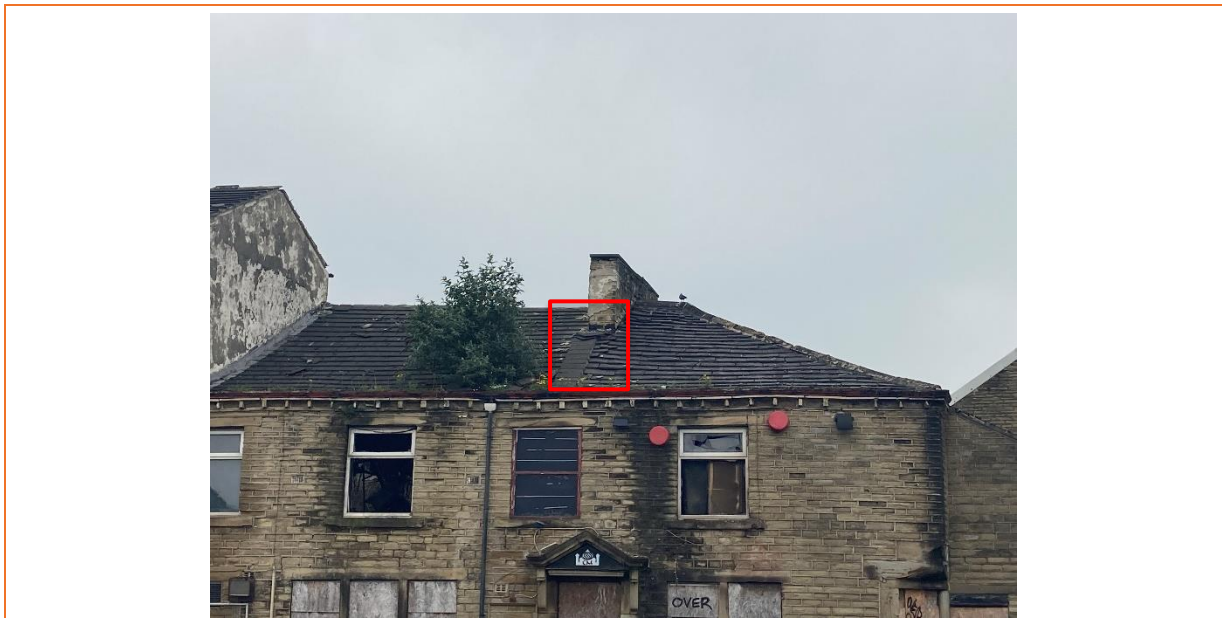
Figure 15 Showing lifted tiles below the stone feature (PRF 12)
