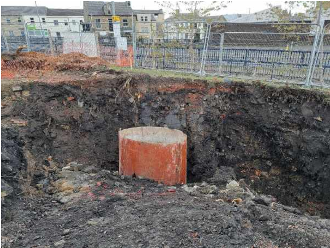
Photograph 4 Red shoring depicts approximate location of encountered shaft on the south-eastern boundary.
