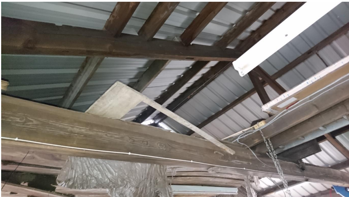
Figure 5: One of two trusses in the workshop missing a queen post
