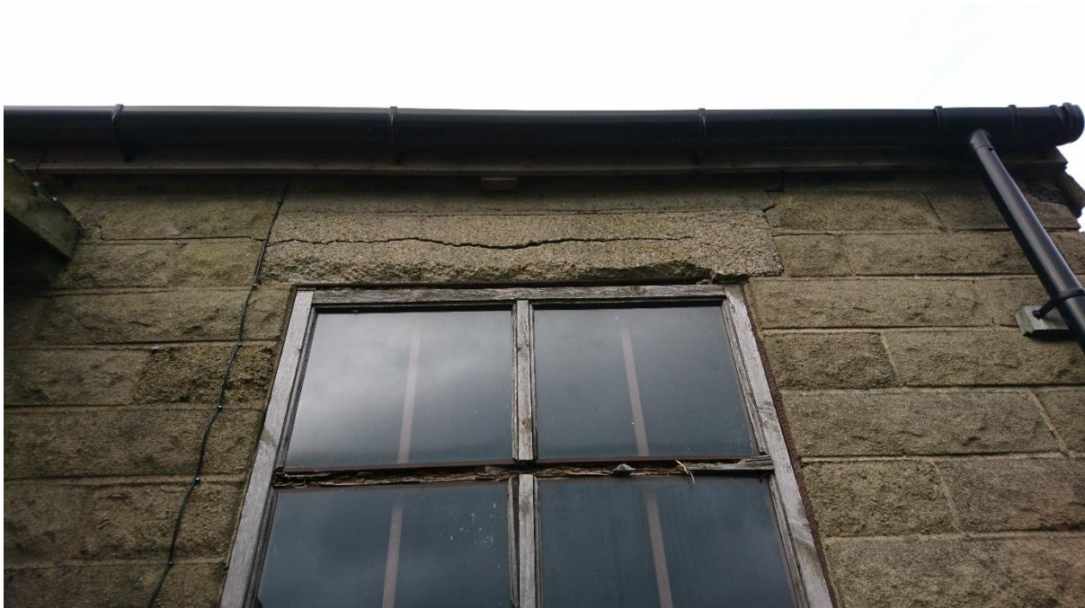
Figure 13: Cracking to the masonry and lintels in the south-eastern elevation, noting the rainwater downpipe to image RIGHT.
