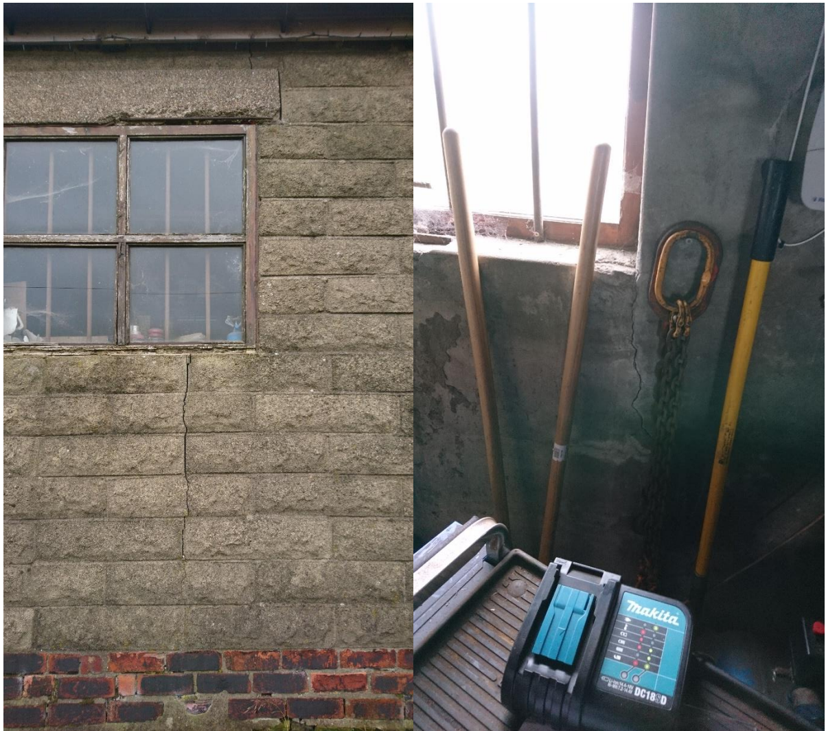
Figure 11: Internal and external tapering cracks in the north-western elevation
