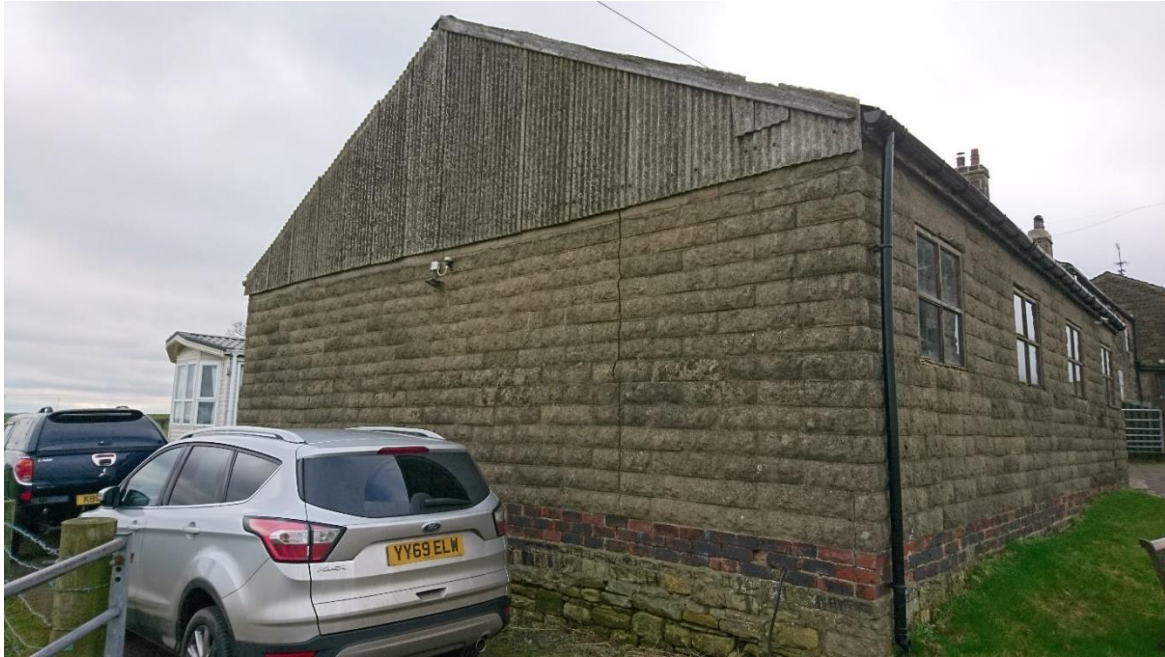
Figure 7: External view of the north-eastern gable, noting tapering cracks.
