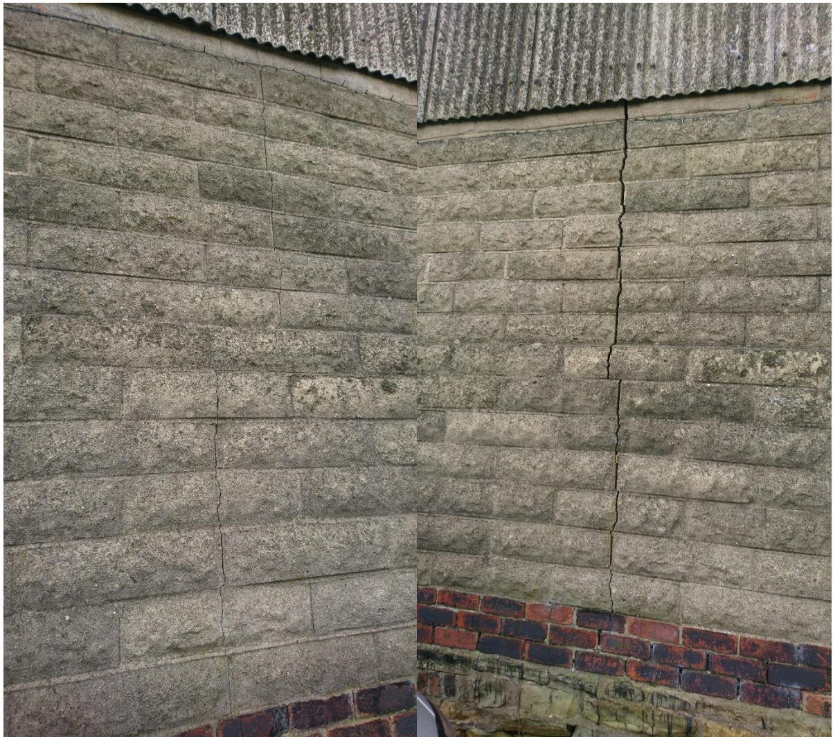
Figure 8: Detail view of the tapering cracks in the north-eastern gable
