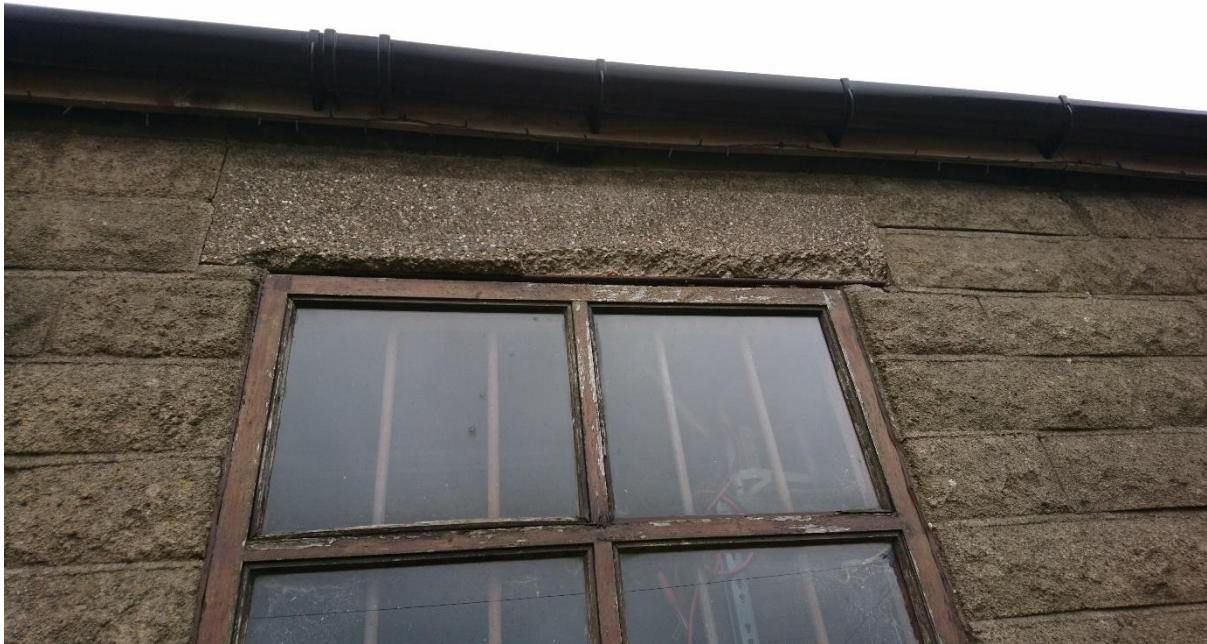
Figure 12: Loss of cover to the cast in-situ concrete lintels.
