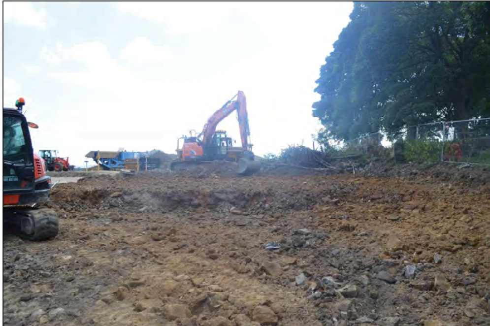
Plate 7. Ground reduction of a house plot in the western edge of the site, looking south
