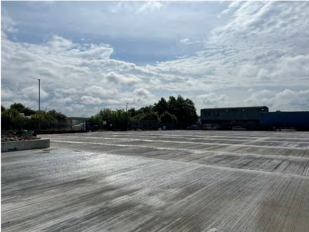
Photograph No.8: View of site from north west corner facing south east.
