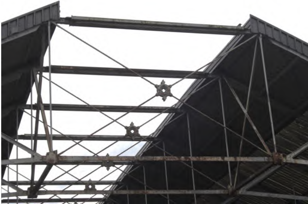
Plate 14: Central cross brace with moulded roundel (or 'rose' connection) and space above marking the location of the former roof lantern
