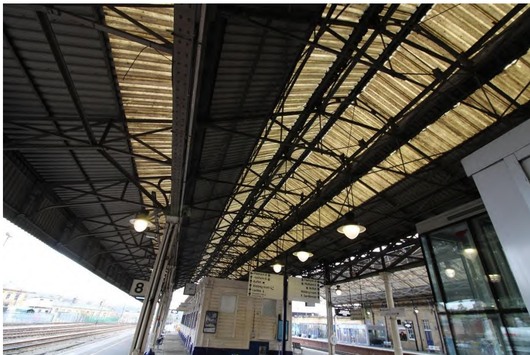
Plate 67: Northern end of Roof B with two station clocks hung either side of the 'Tea Rooms' and three central pendant industrial lights, facing north-east
