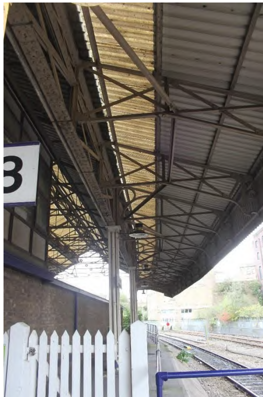
Plate 70: Southern end of Roof C with partial eastern elevation of the Large Brick Warehouse (NHLE 1228533) (right), facing south
