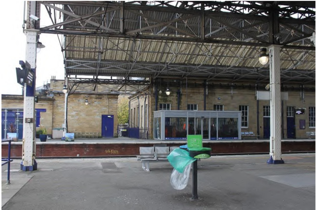
Plate 58: Eastern elevation of two wrought iron columns with lattice beams located at the northern end of Roof B, facing east
