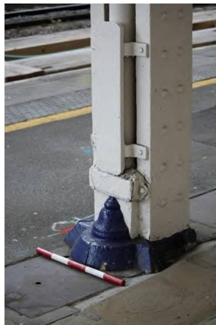
Plate 37: Bell-shaped foot detailing at the base of a compound-riveted wrought iron column with 0.5m scale
