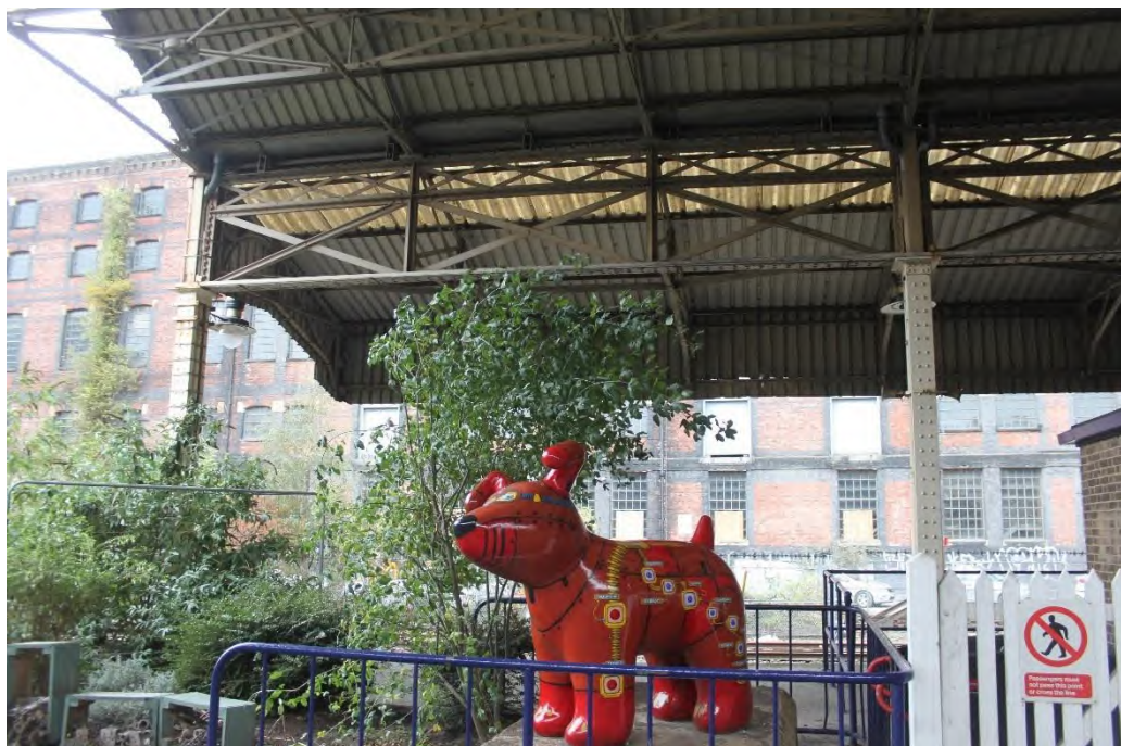
Plate 62: Southern end of western elevation with Large Brick Warehouse (NHLE 1228533) behind, facing west
