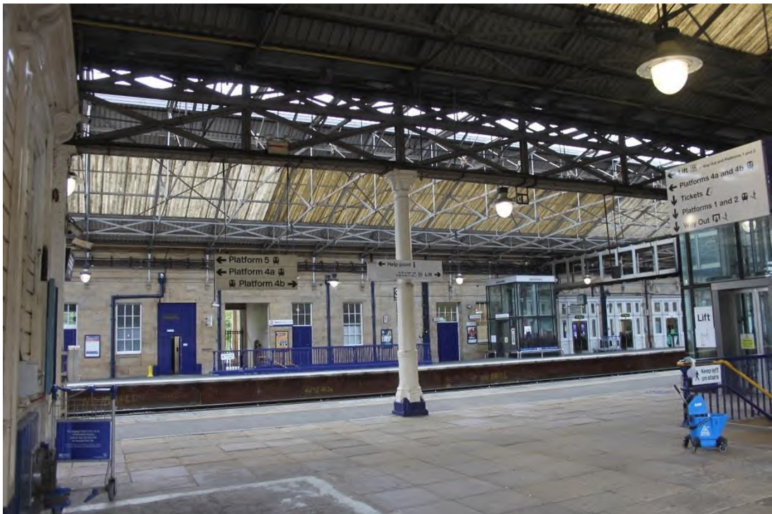
Plate 59: Eastern elevation showing centre-north located cast iron column with lattice beams above, facing east
