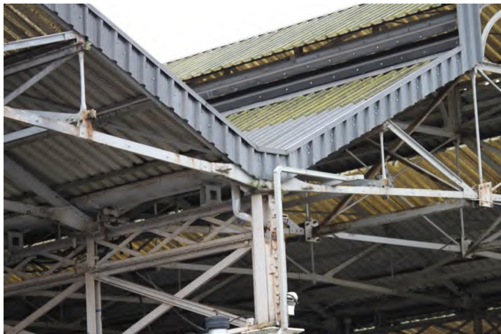
Plate 50: Northern corner of eastern elevation showing longitudinal slats and translucent corrugated fibre pitched roof of lantern with attached western corner of Roof A (centre-left), facing south-west
