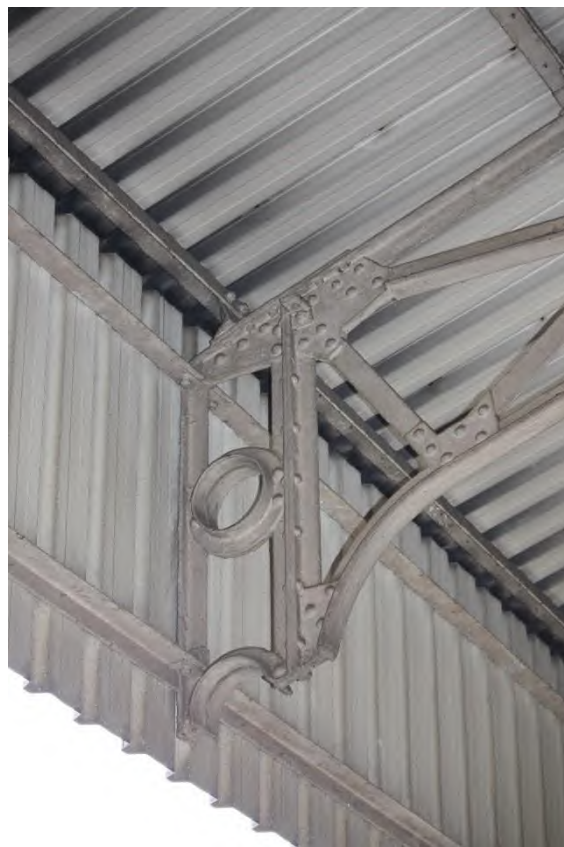
Plate 72: Example of the western end of a riveted lattice wrought iron bracket attached to the western dropdown corrugated metal sheeting
