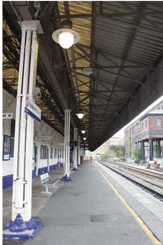
Plate 52: Lower western elevation of Roof B with Large Brick Warehouse (NHLE 1228533) (far-right) facing south
