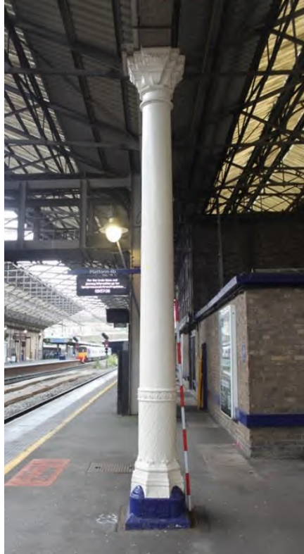
Plate 38: One of the two decorative cast iron columns with 2m scale, facing south
