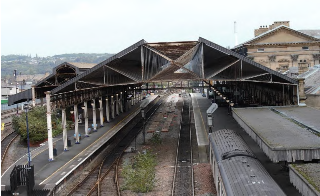
Plate 21: Southern end of Roof A with Roof B and Roof C (far left), Huddersfield Station (NHLE 1277385) (right) and Penistone Line canopy (bottom-right), facing north
