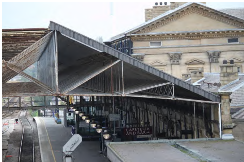
Plate 24: Eastern end of truss attached to the western elevation of the sandstone wall (far right) with the Penistone Line canopy attached (bottom right) and Huddersfield Station (NHLE 1277385), facing north-east
