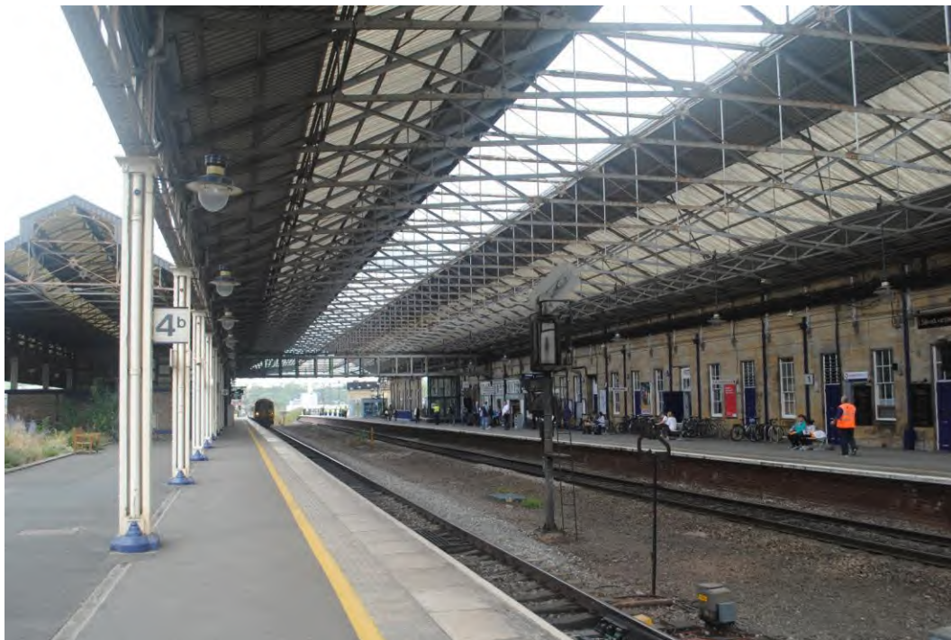
Insert 4-4 Trainshed roof at Huddersfield Station, viewed from southern end of island platform; the main span of ‘Roof A’ is in the foreground while the smaller secondary ‘Roof B’ span can be seen on the left.
