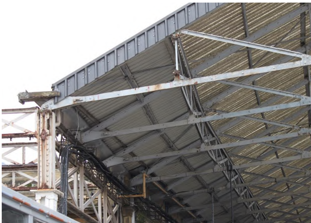
Plate 16: Eastern corner of Roof A on top of a cast iron support
