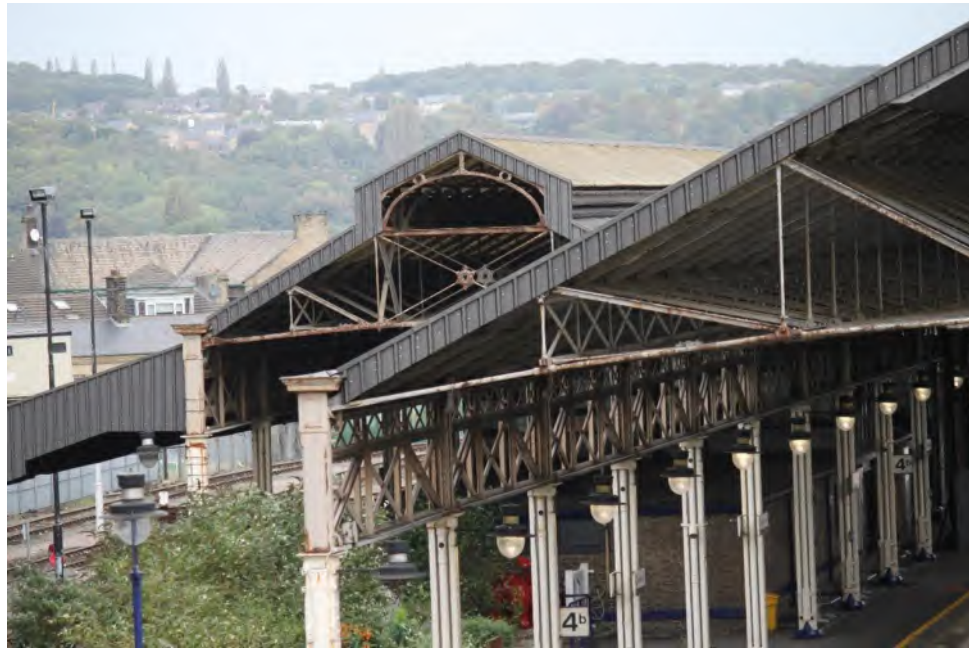
Plate 23: Western column with eaves trough above (centre-left) with the same present on the western side of Roof B (left)
