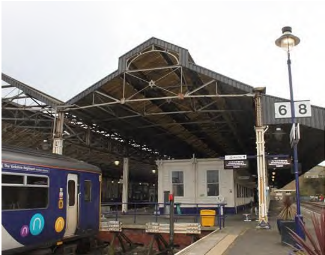
Plate 45: Northern gable end of Roof B with attached Roof A (left) and Roof C (right) and Tea Rooms (centre-right), facing south-east
