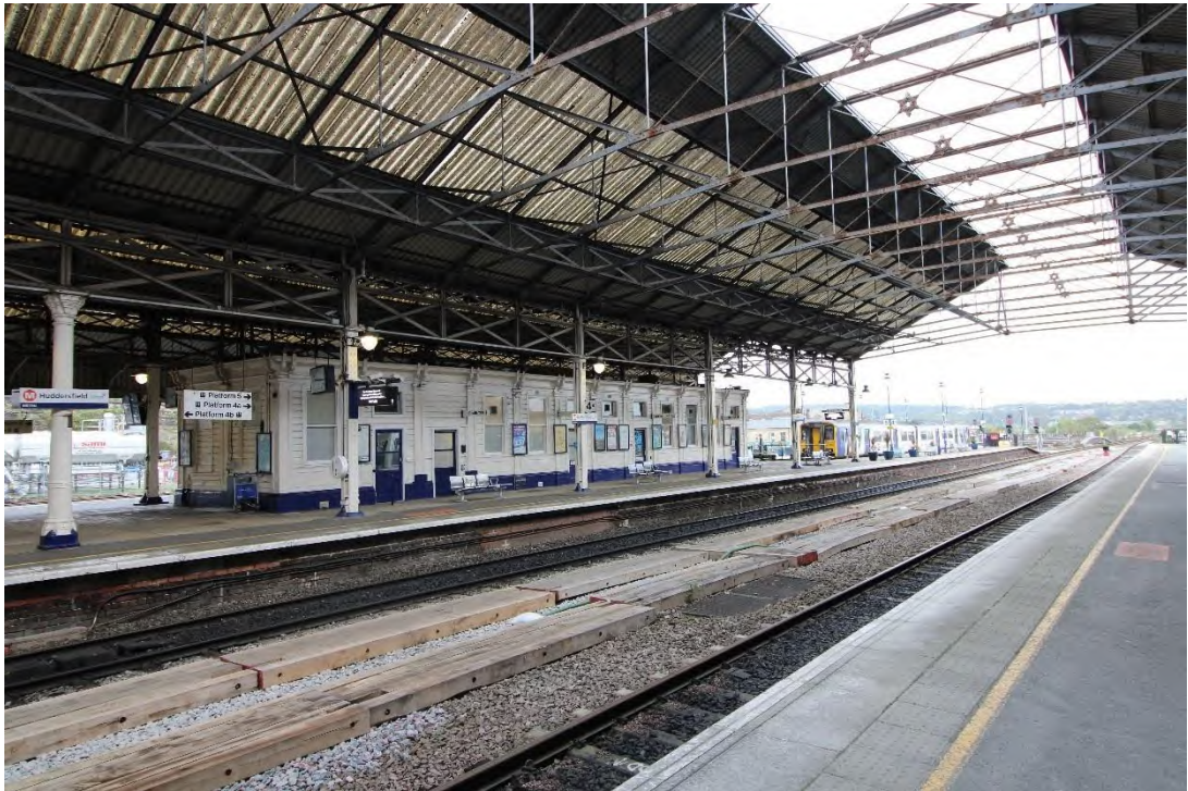
Plate 33: Northern end of western elevation with the eastern elevation of the 'Tea Rooms' located at the northern end of the island platform, facing north-west
