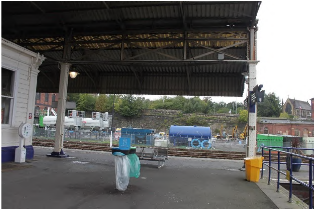
Plate 61: Western elevation of two wrought iron columns with lattice beams located at the northern end of Roof B with the goods yards visible behind, facing west
