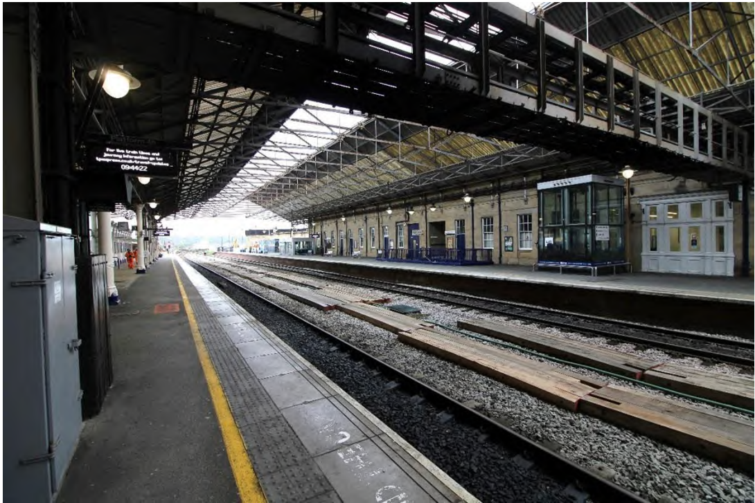
Plate 27: Northern end of eastern elevation (rear (western) elevation) of the station buildings, facing north-east
