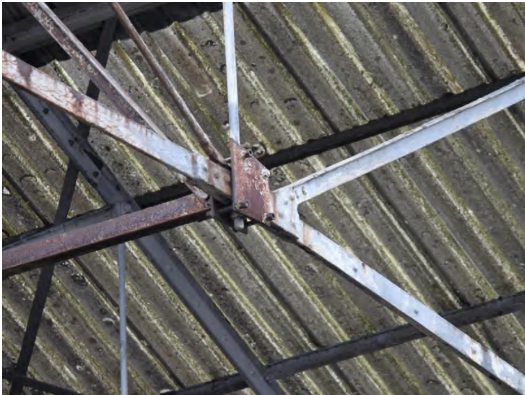
Plate 13: Example of a later join plate attached over an original connection plate at the western end of the northern truss
