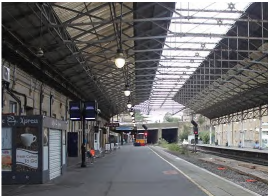
Plate 44: Pendant industrial lighting attached to the western side of the roof trusses
