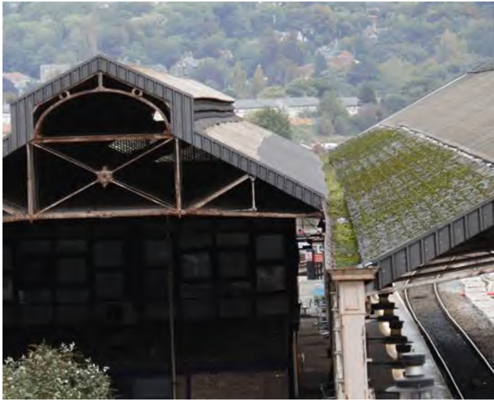
Plate 49: Eastern pitched roof of Roof B (centre) with eastern pitch of roof lantern above (centre-left) and Roof A attached (right), facing north
