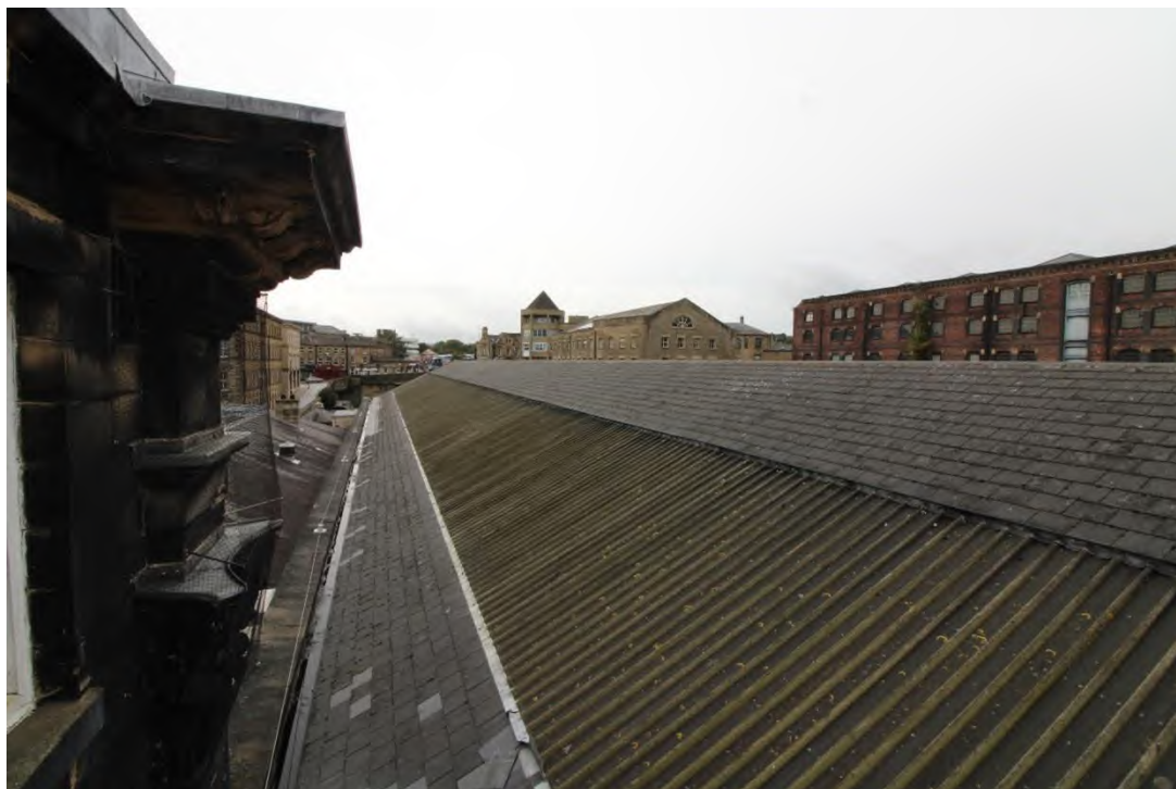
Plate 20: Roof A attached to the rear (western) elevation of the Huddersfield Station and southern wing (NHLE 1277385) (left) with the Large Brick Warehouse (NHLE 1228533) (right) and the Stone Warehouse (NHLE 1287149) (centre)
