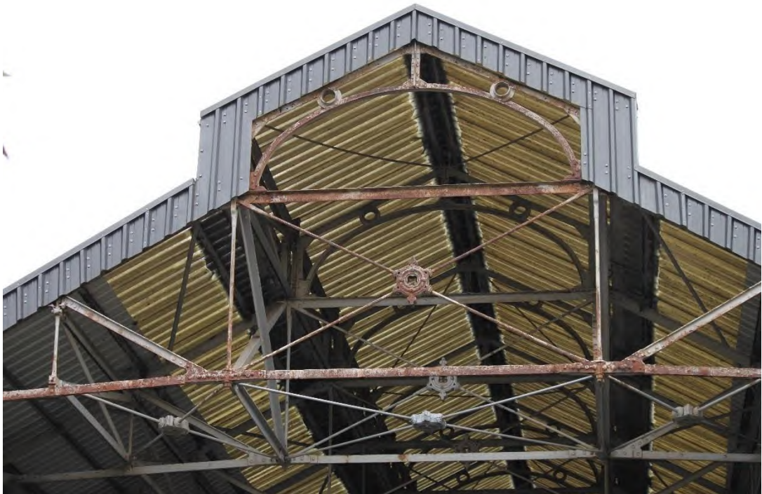
Plate 56: Southern gable end of raised roof lantern with central cross brace and moulded roundel beneath
