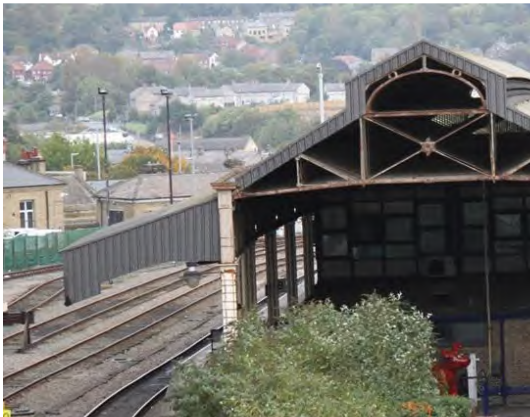
Plate 68: Southern elevation of Roof C (left) attached to western edge of Roof B (centre), with the Former Good Storage Yard and former Office Building visible in the goods yard (background left), facing north
