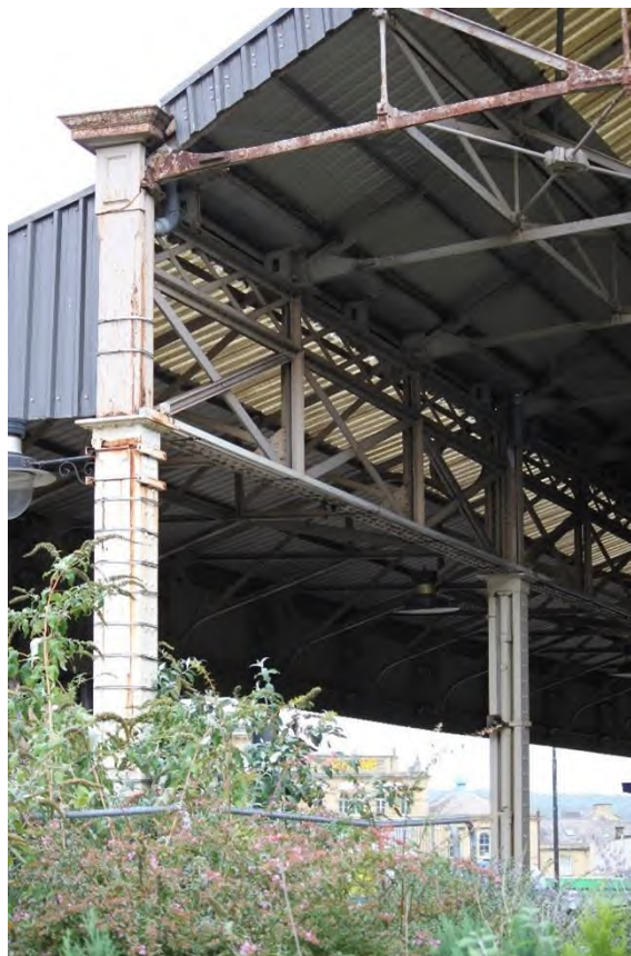
Plate 63: Southern corner of western elevation showing the western ends of the principal trusses connected above the small Howe truss, facing north-west
