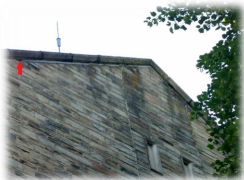
Plate 3: Gap at wallhead.
