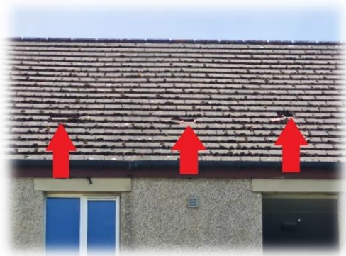
Plate 1: Gaps in roof.
