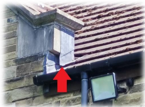
Plate 4: Gap under flashing.
