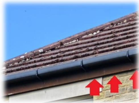
Plate 2: Gaps under fascia.
