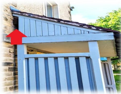
Plate 5: Gap between porch woodwork.
