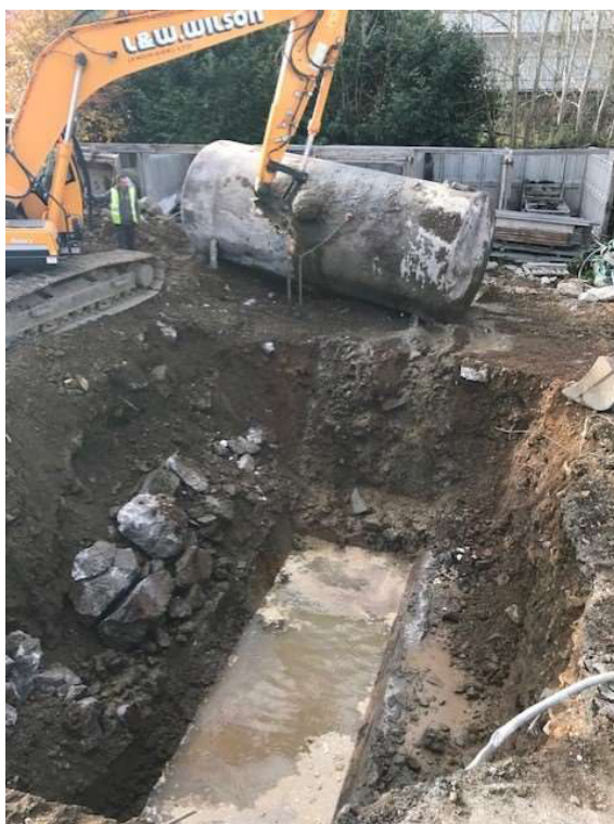
Figure D. Beware of bad practice! A dangerous tank removal in progress with tank contents leaking into the environment after removal.
