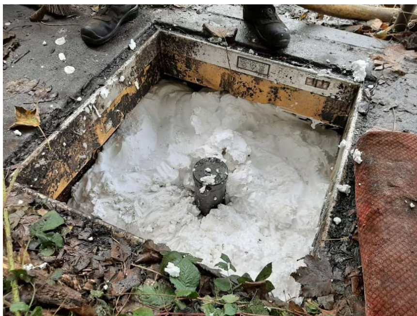
Figure C. A foam filled tank and chamber from the surface.
