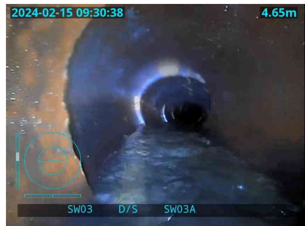
027.jpg, 00:01:07, 4.65 m Open joint, large
