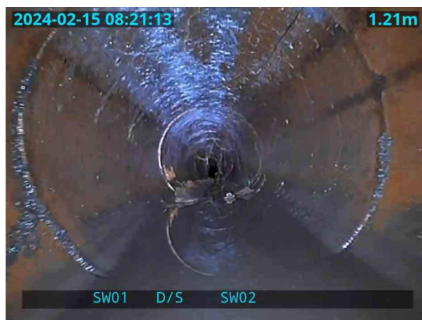
003.jpg, 00:00:20, 1.21 m Roots, fine at joint, start
