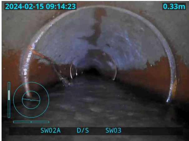
019.jpg, 00:00:12, 0.33 m Roots, fine at joint
