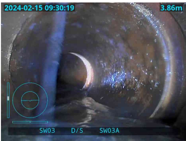
026.jpg, 00:00:48, 3.86 m Open joint, large
