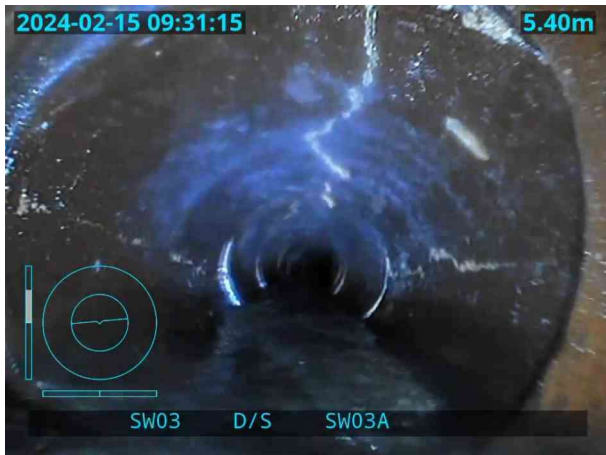
028.jpg, 00:01:44, 5.40 m Fracture, longitudinal at 9 o'clock
