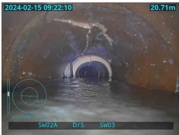
023.jpg, 00:01:45, 20.71 m Fracture, longitudinal at 9 o'clock
