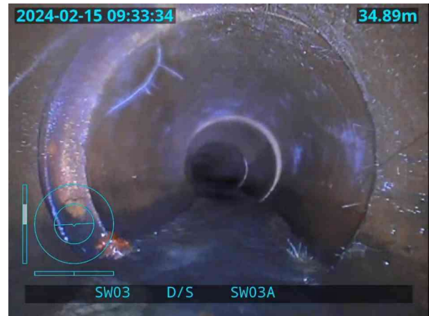
029.jpg, 00:04:03, 34.89 m Open joint, medium
