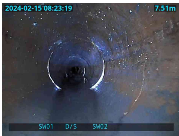
008.jpg, 00:01:38, 7.51 m Fracture, circumferential from 2 o'clock to 6 o'clock
