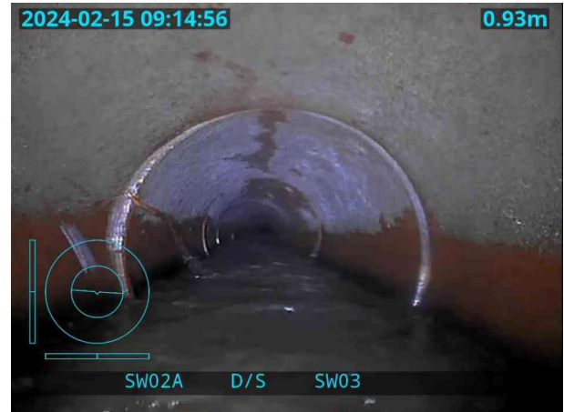
020.jpg, 00:00:44, 0.93 m Survey abandoned, Due to obstruction under water level, poss debris
