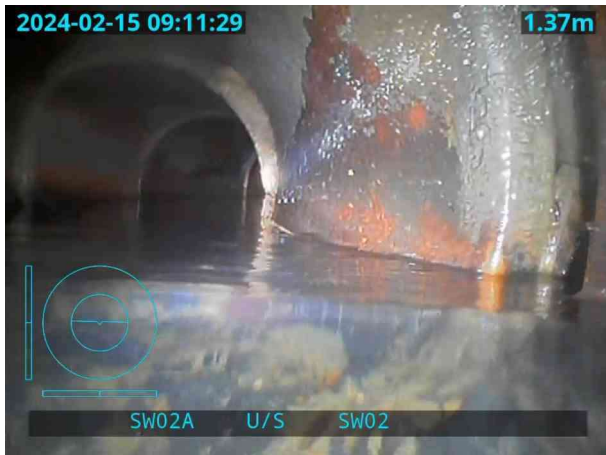
016.jpg, 00:00:18, 1.37 m Open joint, medium
