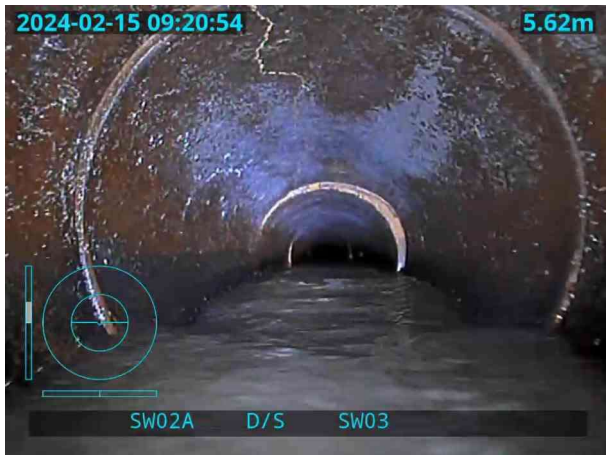
021.jpg, 00:00:29, 5.62 m Crack, longitudinal at joint at 12 o'clock
