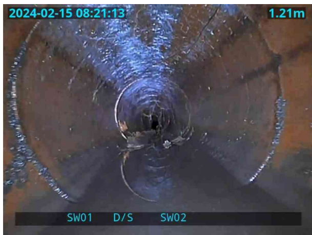
004.jpg, 00:00:20, 1.21 m Fracture, longitudinal at 1 o'clock
