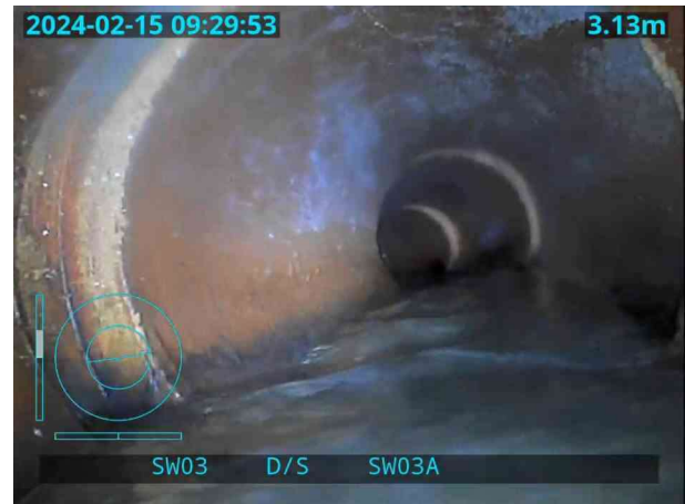
025.jpg, 00:00:22, 3.13 m Open joint, large
