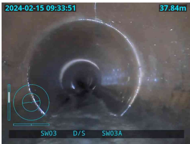
030.jpg, 00:04:20, 37.84 m Crack, longitudinal at 12 o'clock
