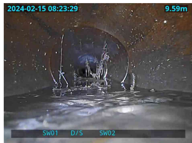
009.jpg, 00:01:49, 9.59 m Settled deposits, fine, 20% cross-sectional area loss, start Under water level
