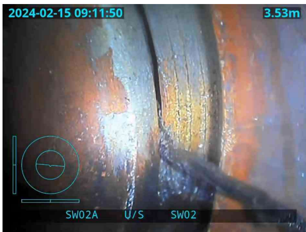
018.jpg, 00:00:39, 3.53 m Roots, fine at joint
