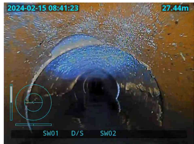
013.jpg, 00:05:16, 27.44 m Broken pipe at joint from 11 o'clock to 12 o'clock
