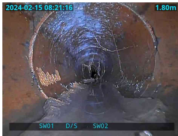
006.jpg, 00:00:23, 1.80 m Settled deposits, fine, 10% cross-sectional area loss
