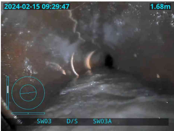
024.jpg, 00:00:16, 1.68 m Fracture, longitudinal at 12 o'clock
