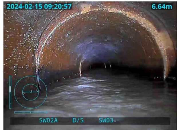
022.jpg, 00:00:33, 6.64 m Joint displaced, medium
