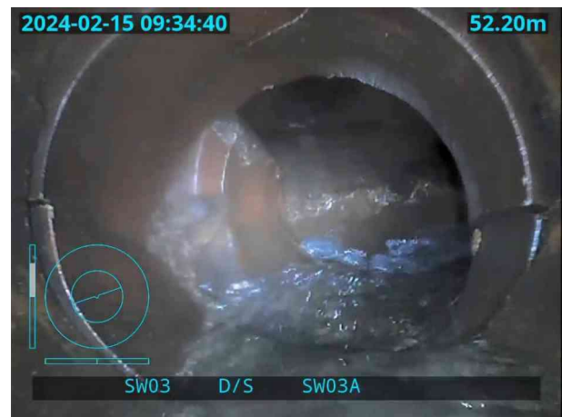
031.jpg, 00:05:09, 52.20 m Fracture, longitudinal at 9 o'clock
