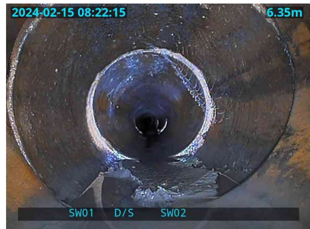
007.jpg, 00:01:22, 6.35 m Settled deposits, fine, 5% cross-sectional area loss
