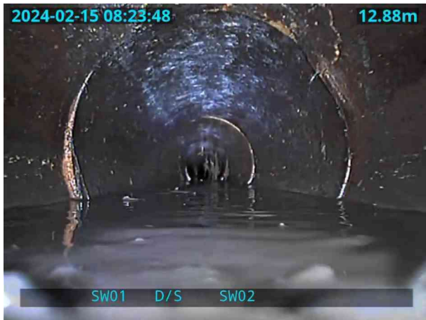
010.jpg, 00:02:07, 12.88 m Fracture, circumferential at joint from 11 o'clock to 2 o'clock
