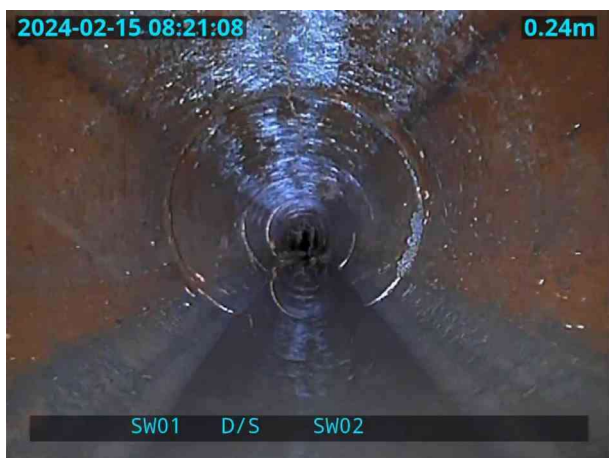
002.jpg, 00:00:15, 0.24 m Fracture, longitudinal at 12 o'clock
