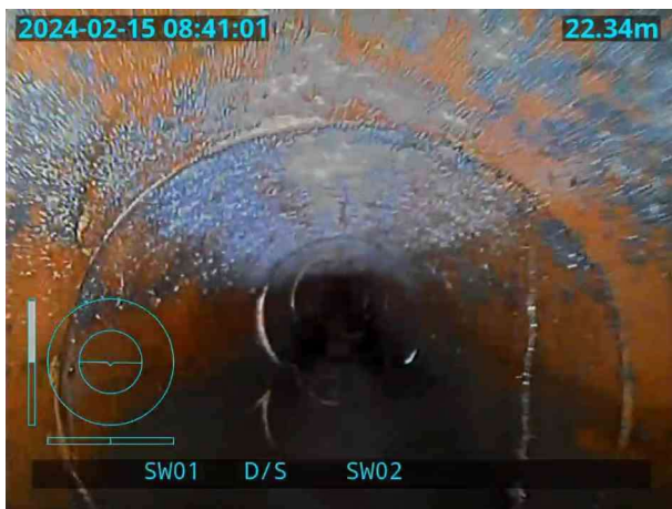
014.jpg, 00:04:54, 22.34 m Crack, circumferential at joint from 10 o'clock to 1 o'clock
