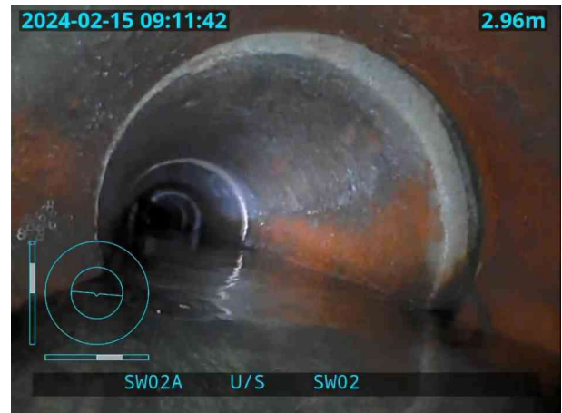
017.jpg, 00:00:31, 2.96 m Joint displaced, medium
