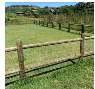
1.1m Galvanised Wire Mesh Fencing incl. electric pasture tape to Pig's Enclosure
