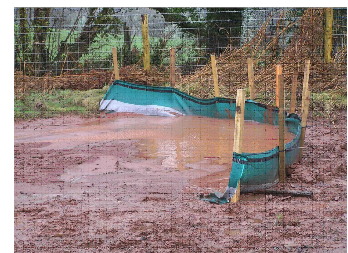
HY-TEX TERRASTOP SILT FENCING TO BE INSTALLED TO MANUFACTURERS SPECIFICATION (Refer to manufacturers installation guidance)
