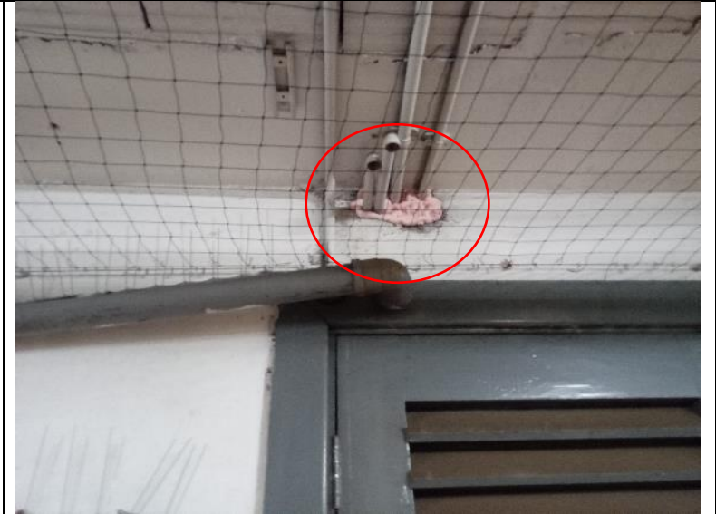
Figure 28. Basement – supporting wall crevices infilled.
