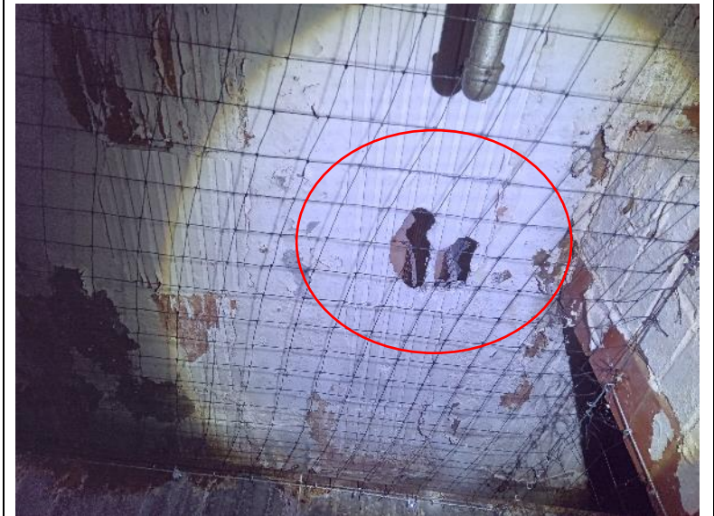
Figure 29. Basement – crevice/cavity in ceiling.
