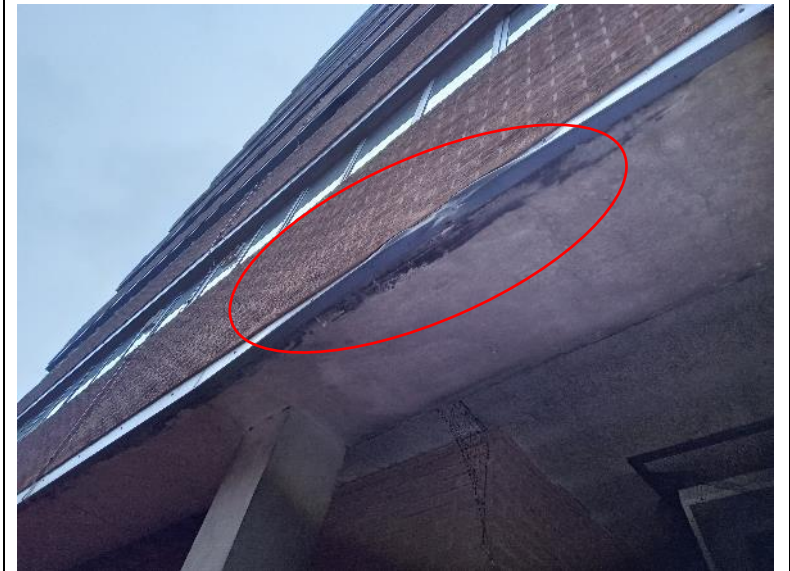
Figure 9. Northern elevation – cosmetic damage.
