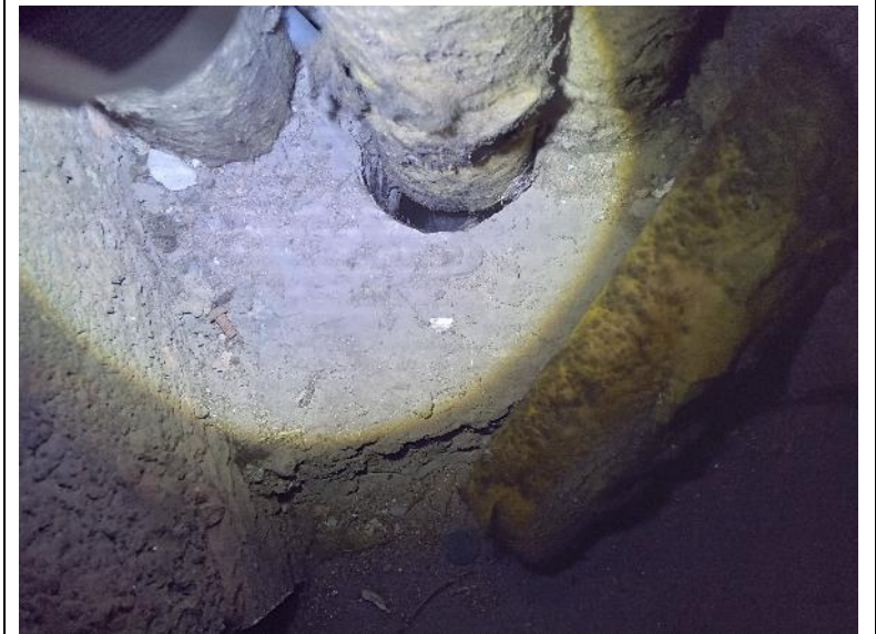
Figure 25. Roof space 2 – gap associated with pipe.
