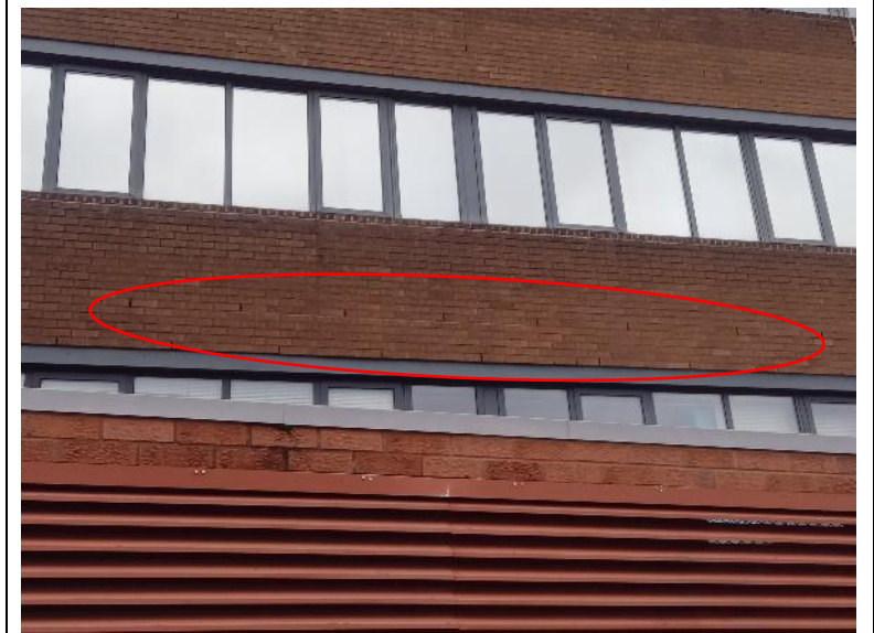
Figure 13. Southern elevation – superficial gaps.
