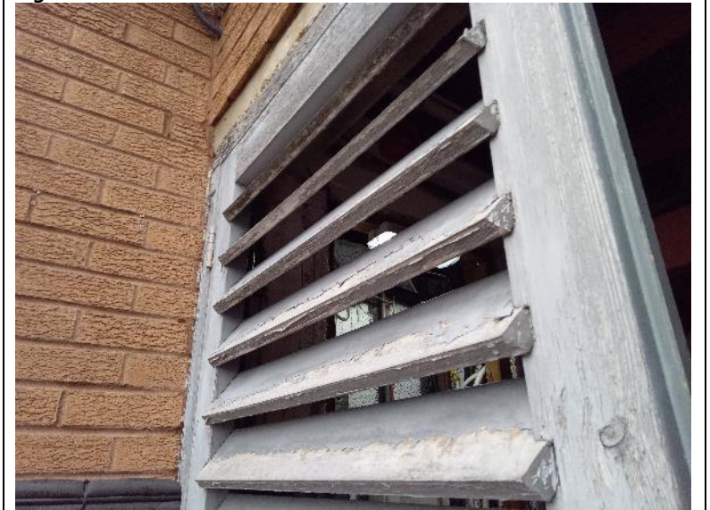
Figure 19. Gaps between shutters on the doors.
