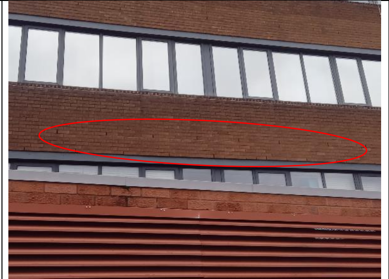
Figure 13. Southern elevation – superficial gaps.
