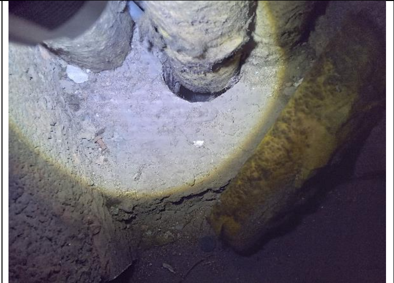
Figure 25. Roof space 2 – gap associated with pipe.
