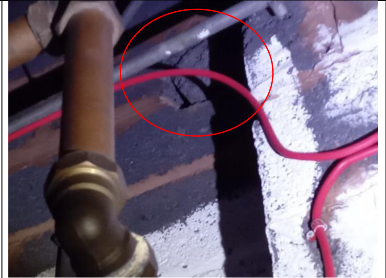
Figure 21. Roof space 1 – crevice.
