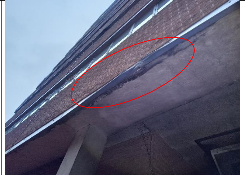
Figure 9. Northern elevation – cosmetic damage.
