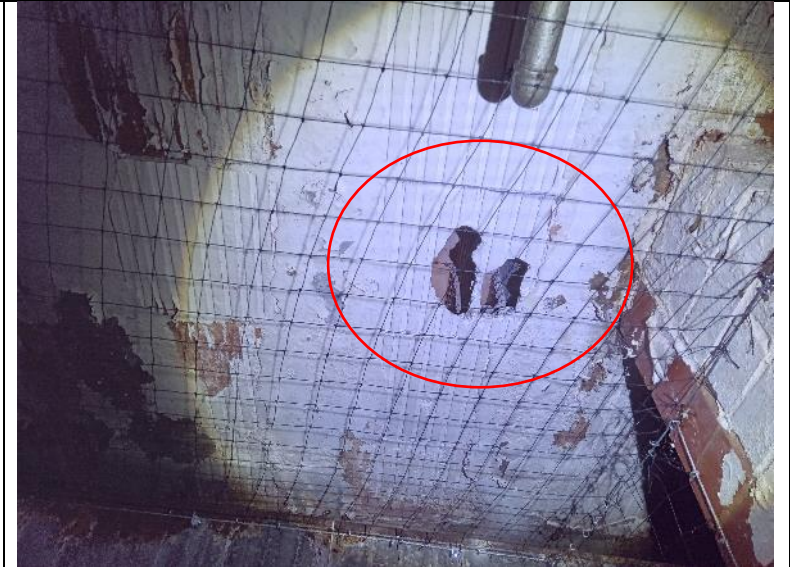
Figure 29. Basement – crevice/cavity in ceiling.
