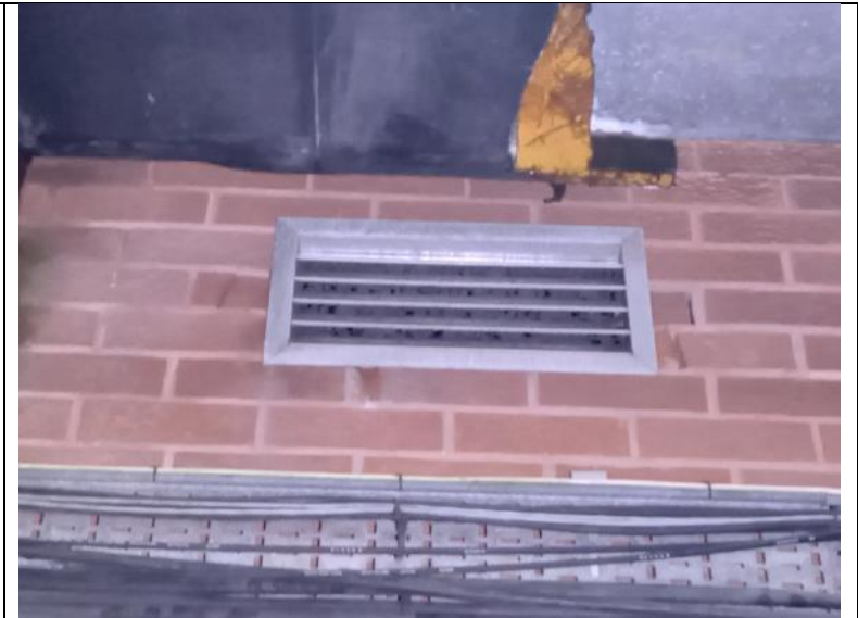
Figure 11. Western elevation – sealed vent.
