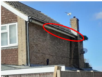
Image 05: Gap between wall top and roof on eastern elevation and lifted tile at base of chimney
