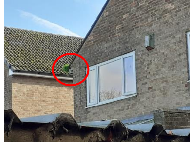
Image 02: Missing soffit end cap
