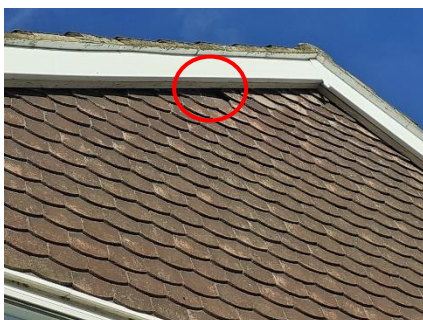
Image 07: Missing hanging tile on southern elevation
