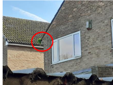
Image 02: Missing soffit end cap
