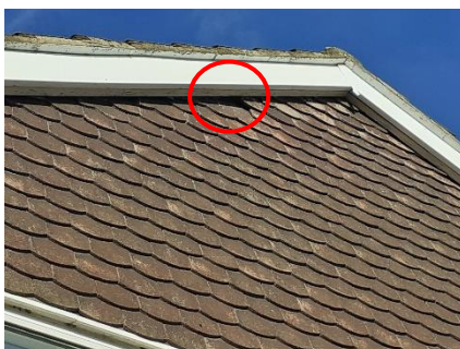
Image 07: Missing hanging tile on southern elevation
