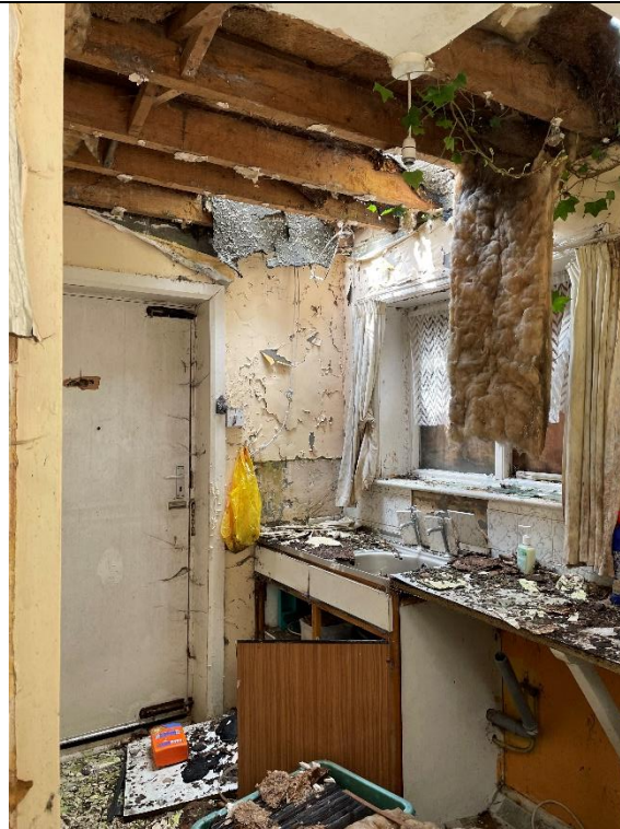
GF side kitchen – roof collapse above
