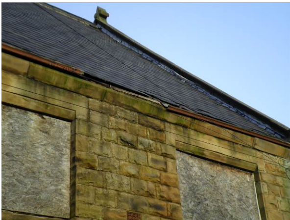
Photo 3 Rotten eaves gutter
