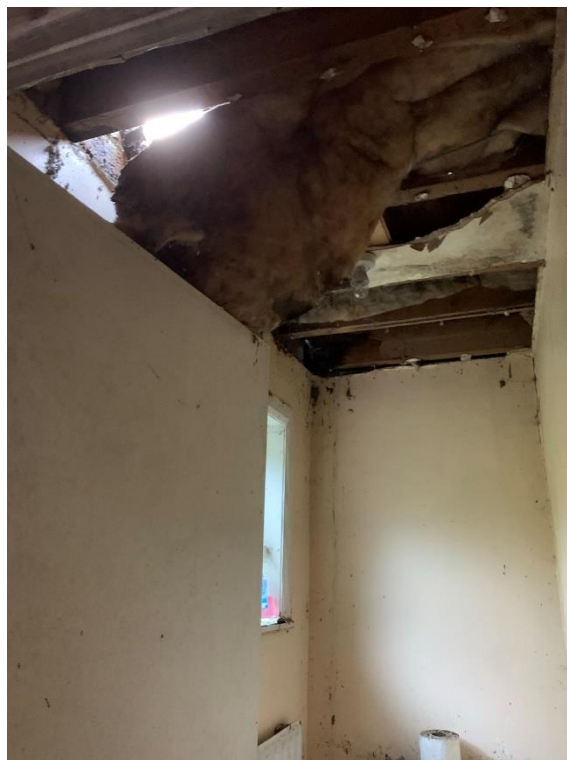
GF toilet roof collapse
