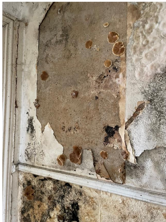
General dampness and water ingress at FF
