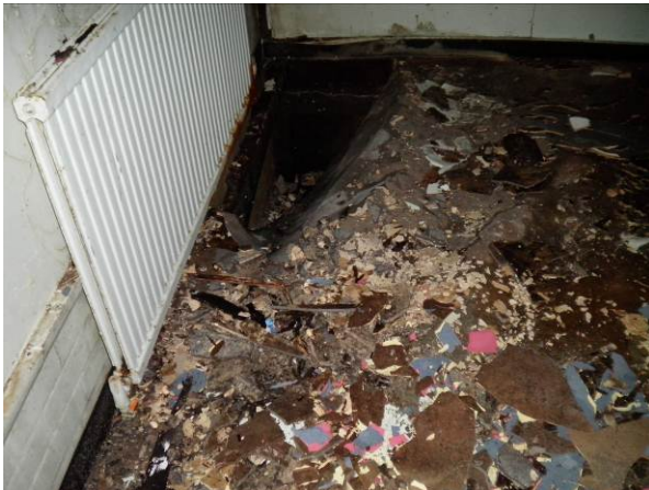
Photo 15 Rotten and collapsed floor
