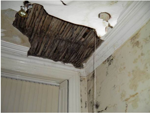
Photo 5 Damaged ceiling and water ingress to 1 st floor
