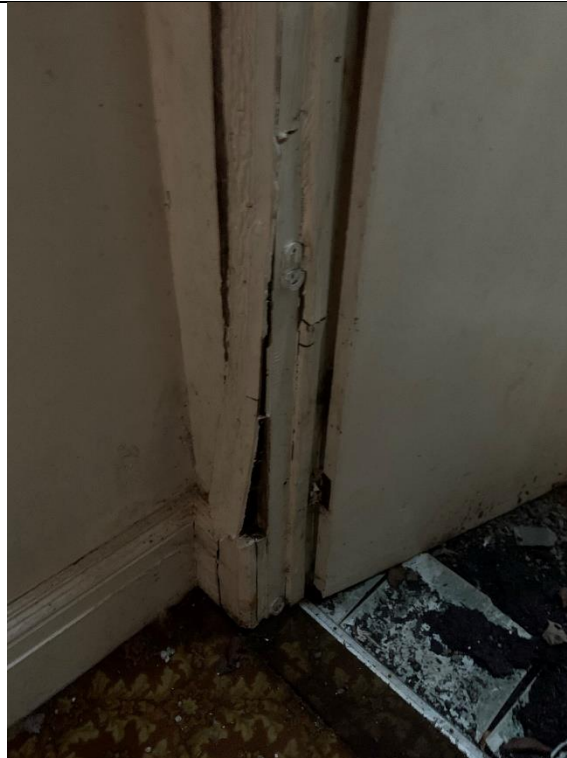
Typical wet rot to GF joinery
