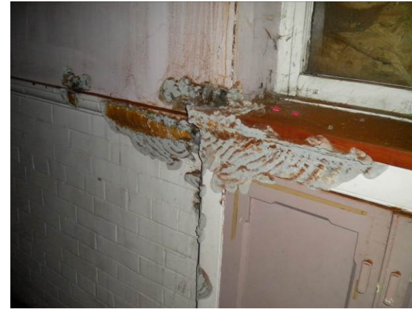
Photo 14 Dry rot to window reveal, cill and built-in cupboard
