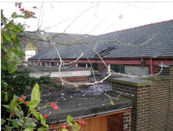
Photo 3 Overall view of defective pitched and flat roofs
