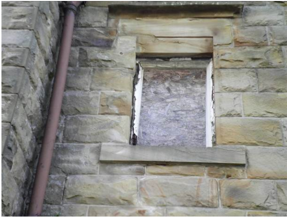
Photo 5 Typical example of rotten window frame
