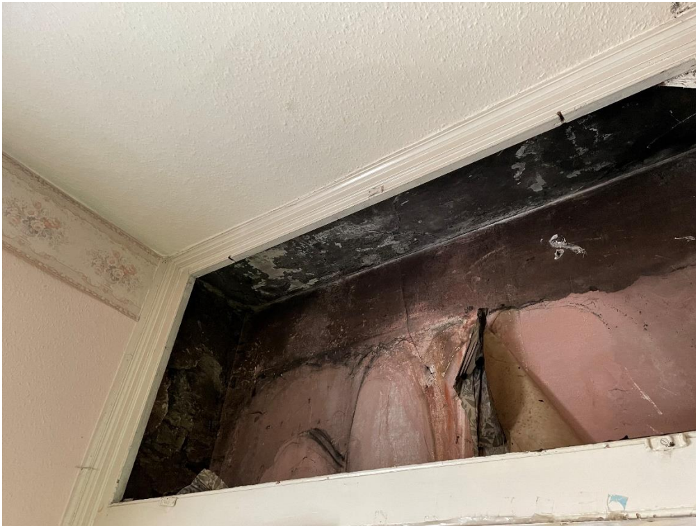
General dampness and water ingress at FF
