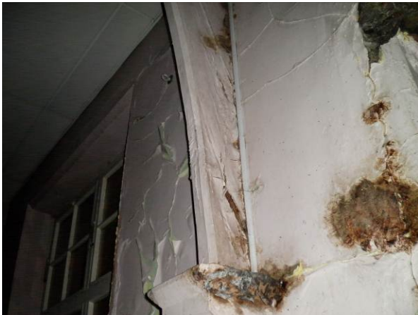
Photo 11 Rotten timber to truss member
