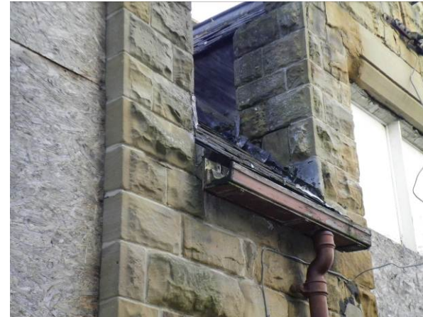
Photo 2 Defective roof and gutter. Missing lead flashings and sheeting to dormer cheek.
