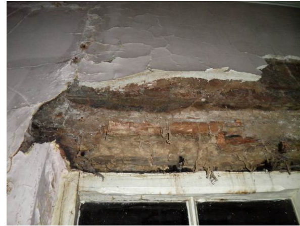
Photo 10 Rotten timber beam
