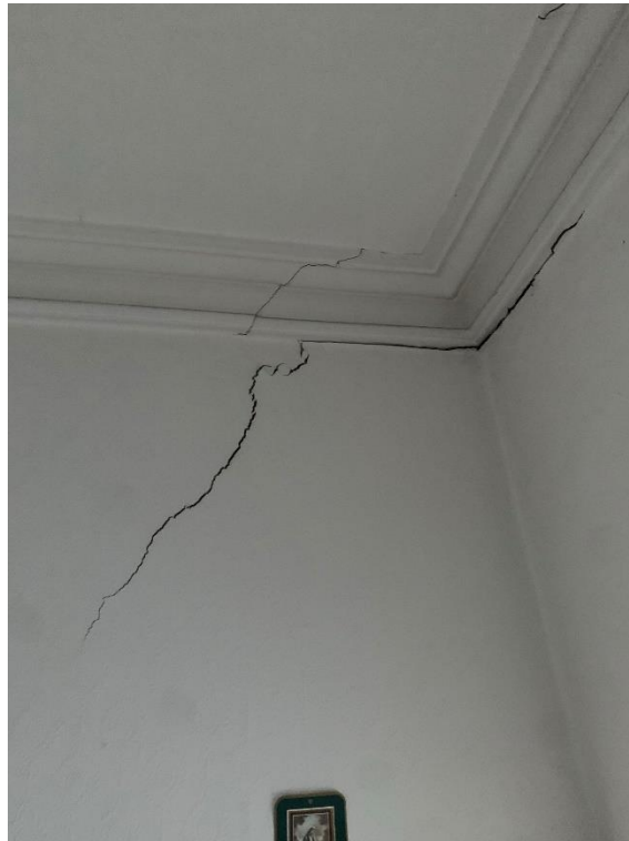
FF cracking and movement to side gable
