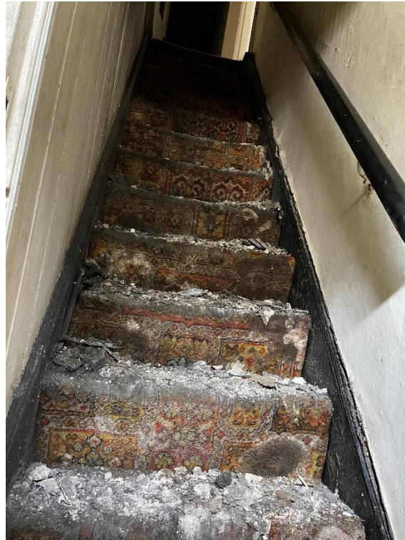
General poor condition of staircase
