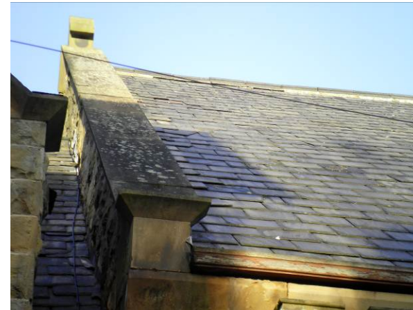
Photo 2 Defective slating to main roof
