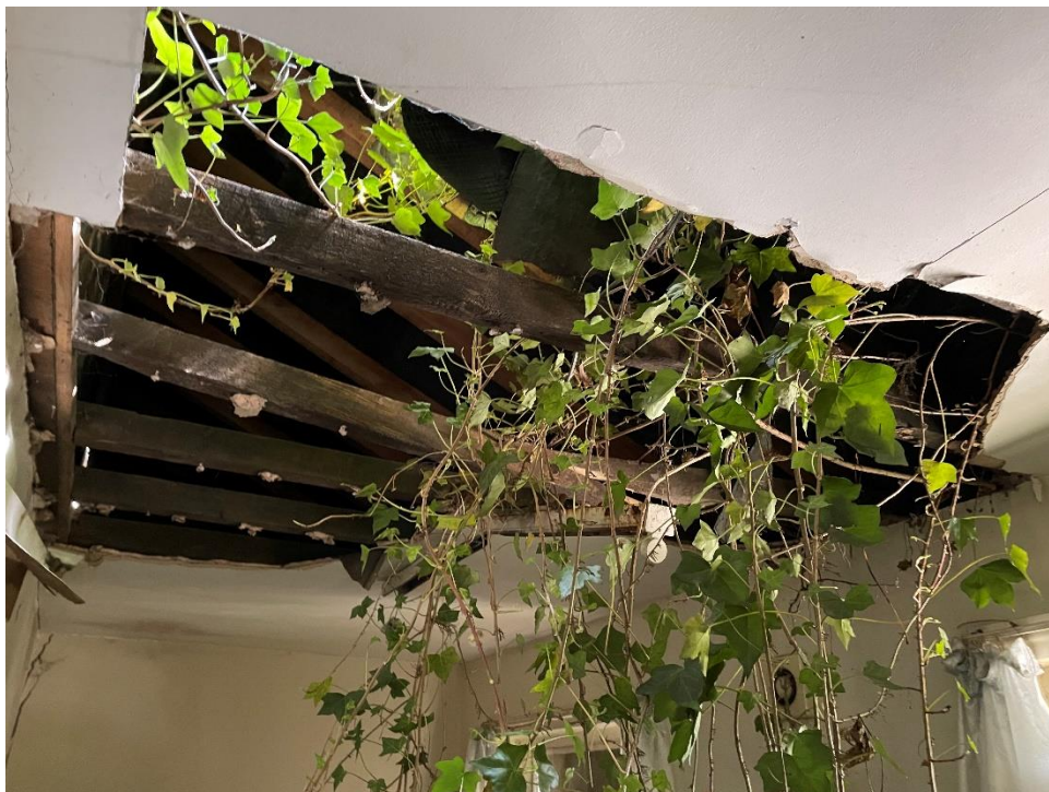
GF rear kitchen roof structure collapse
