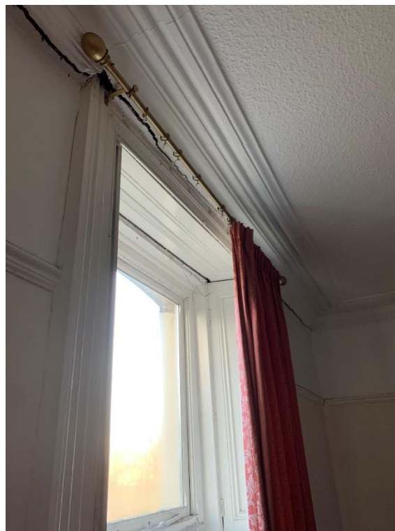
Further GF movement to front elevation
