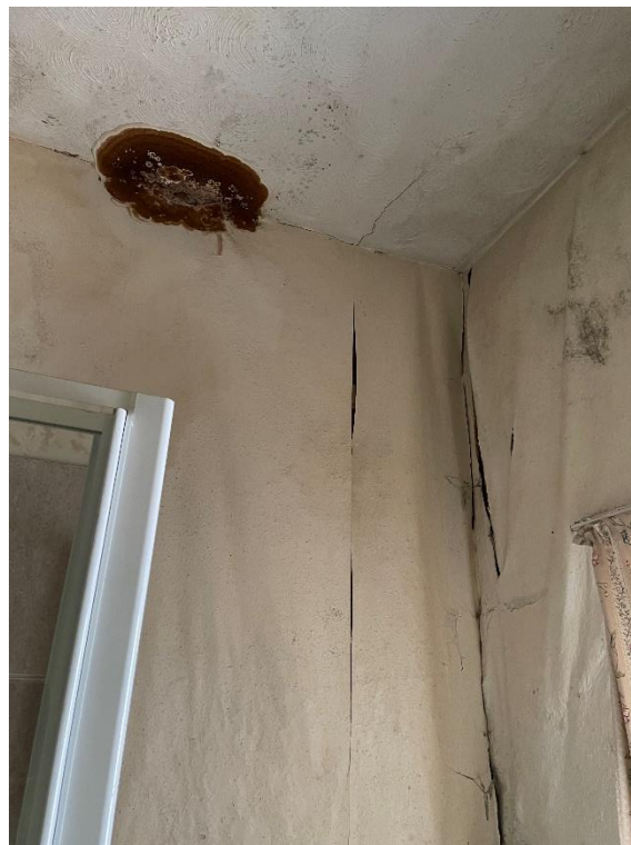
General dampness and water ingress at FF
