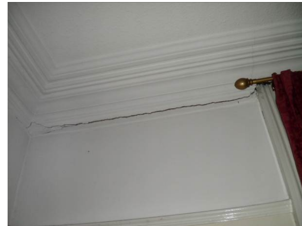
Photo 4 Typical internal cracking
