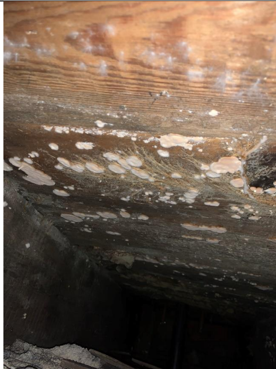
Wet rot to GF floor structure – taken from basement
