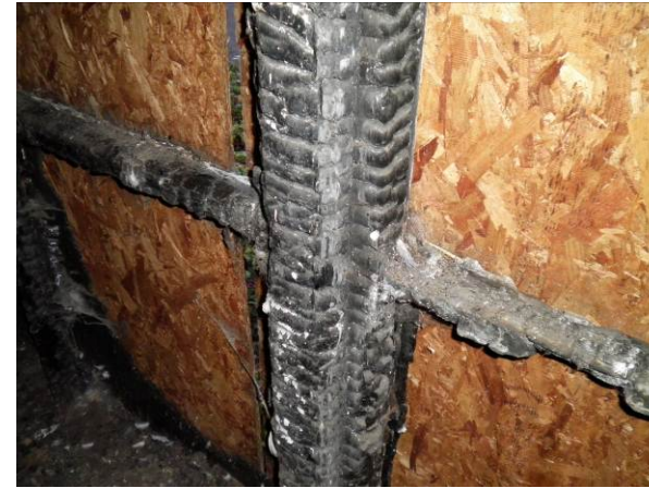
Photo 6 Typical fire damage to external timber framing
