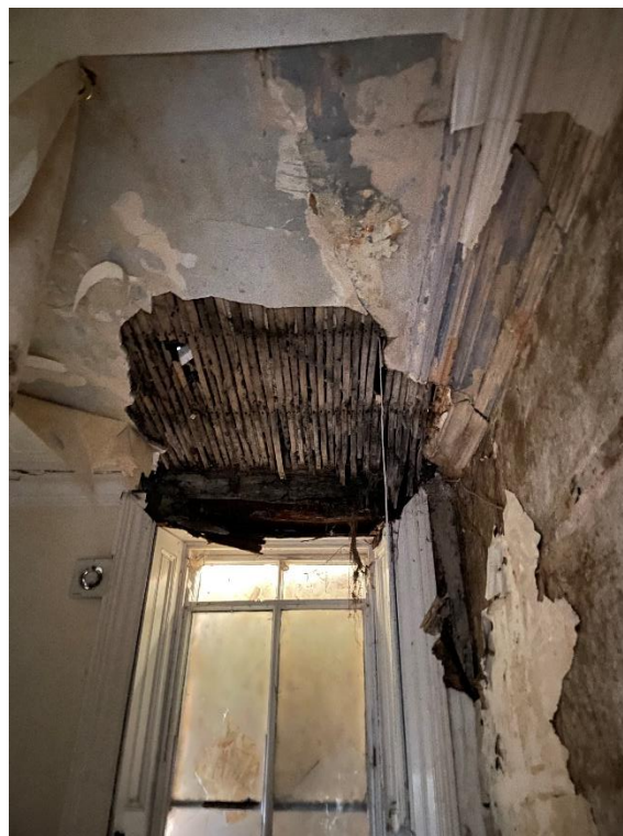
Ground floor ceiling damage from roof level water ingress
