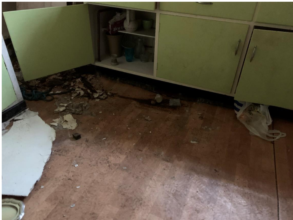
GF main kitchen floor slab sunk and rotated
