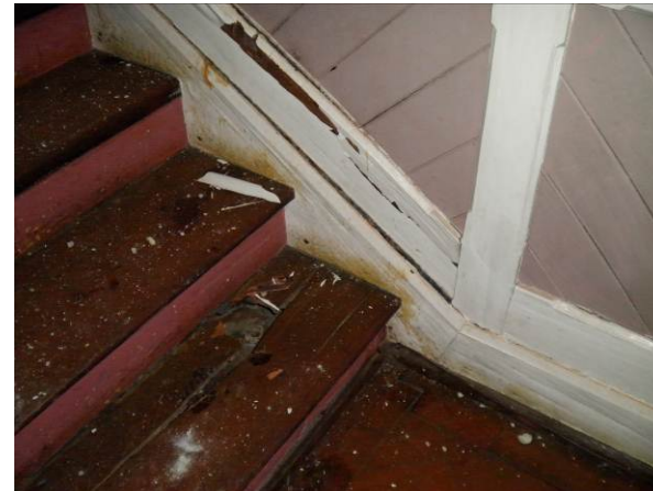
Photo 12 Dry rot to stairs
