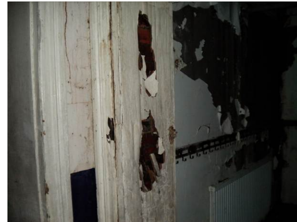
Photo 16 Rotten door frame and water ingress
