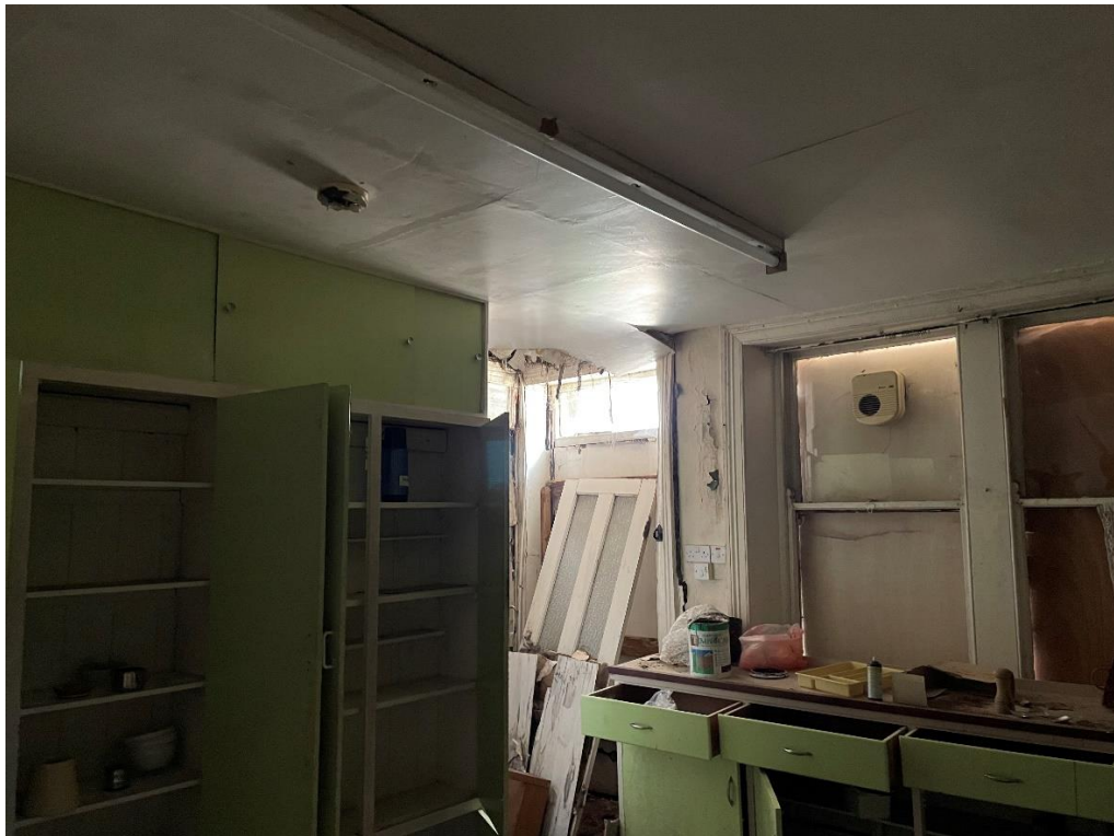
GF Kitchen damage
