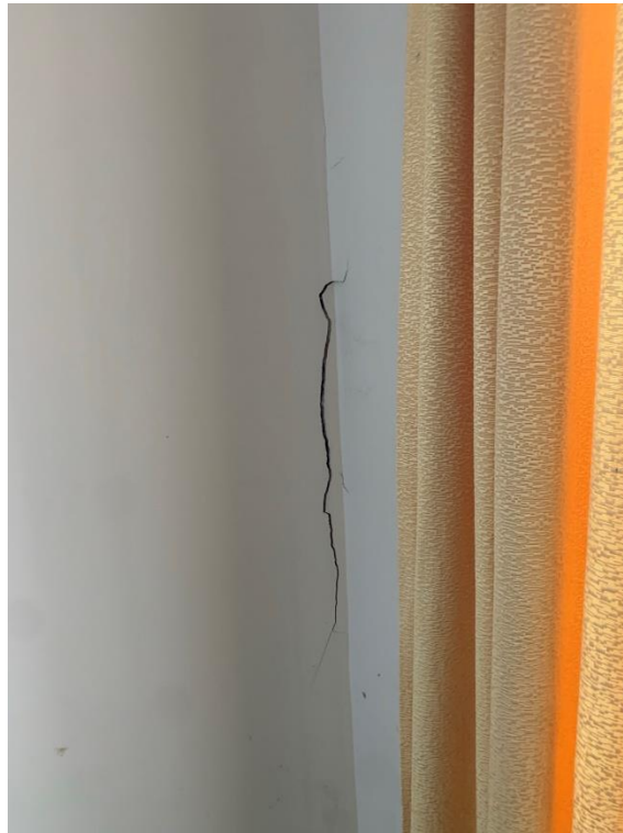
FF cracking to front elevation
