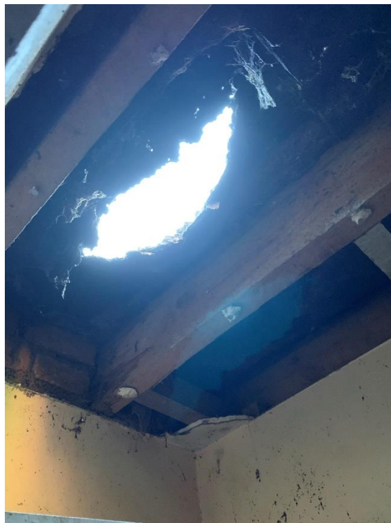
Roof collapse above toilets
