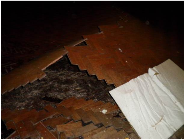
Photo 9 Swollen parquet flooring to main hall
