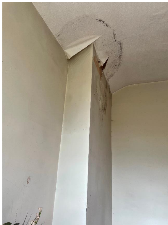
Water ingress around upper chimney
