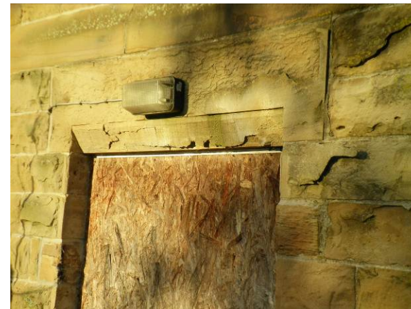
Photo 4 Typical cracking and delaminating stonework
