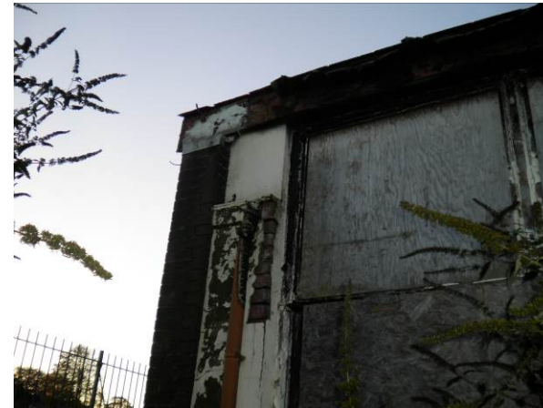
Photo 2 Fire damaged window frame, fascia, melted rainwater goods etc
