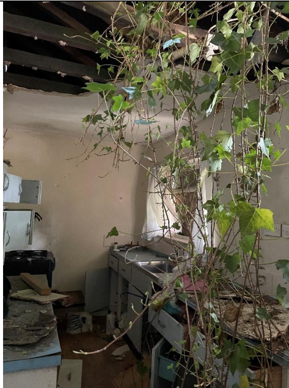
GF rear kitchen damage due to roof structure collapse
