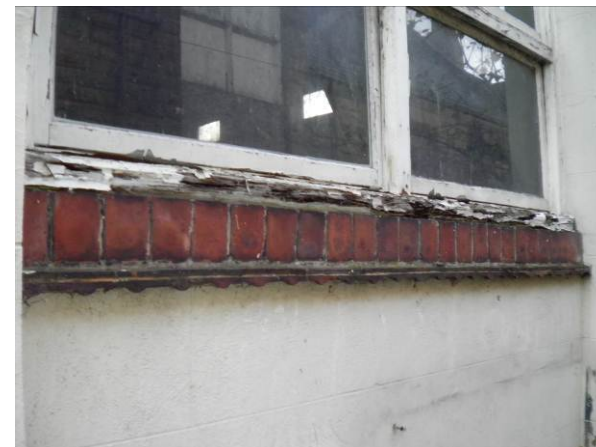
Photo 4 Typical rotten window frame
