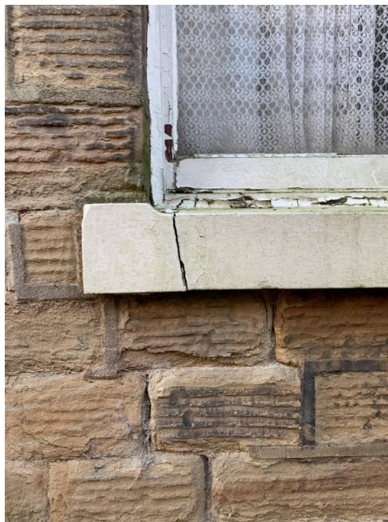
Cracking extending to stone cills
