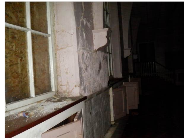
Photo 8 Extent of dampness to external walls
