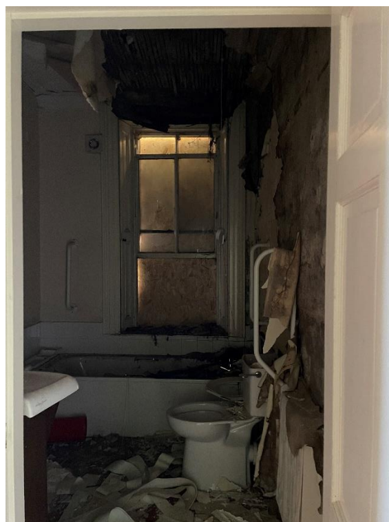
GF Bathroom affected by ceiling collapse and water ingress
