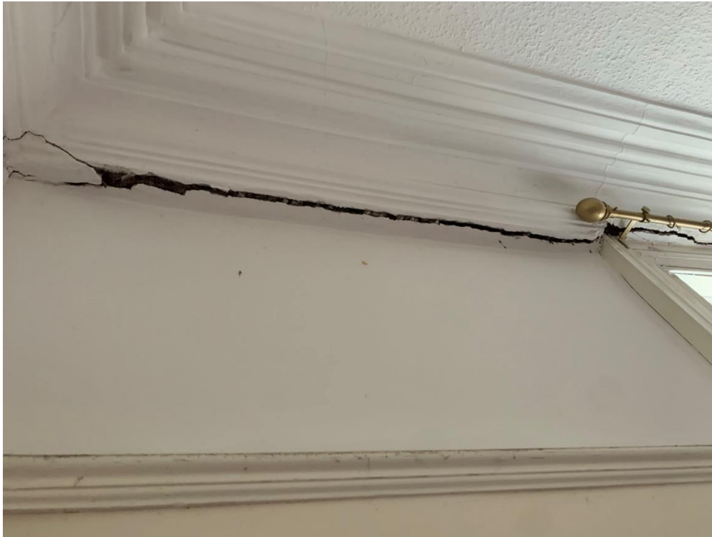
Further GF movement to front elevation
