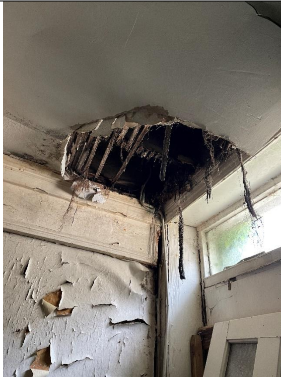
Collapsed ceiling and floor structure above GF main kitchen
