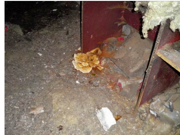
Photo 8 Active dry rot to floor/internal joinery
