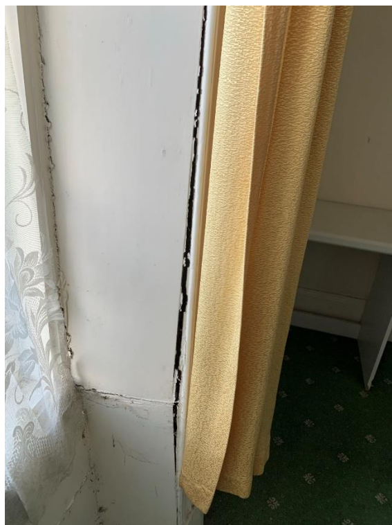
FF cracking and movement to front elevation
