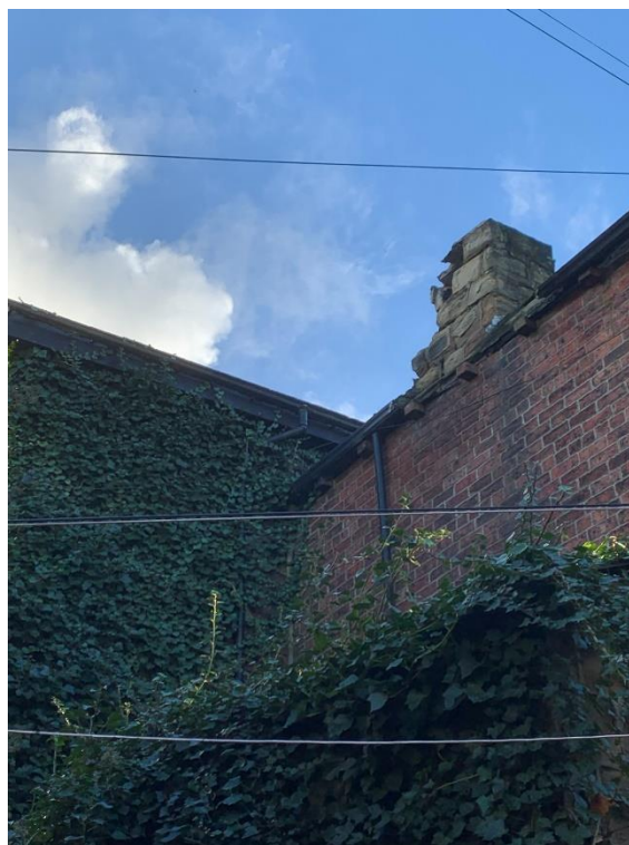
Rear Chimney collapse and gutter and fascia failure
