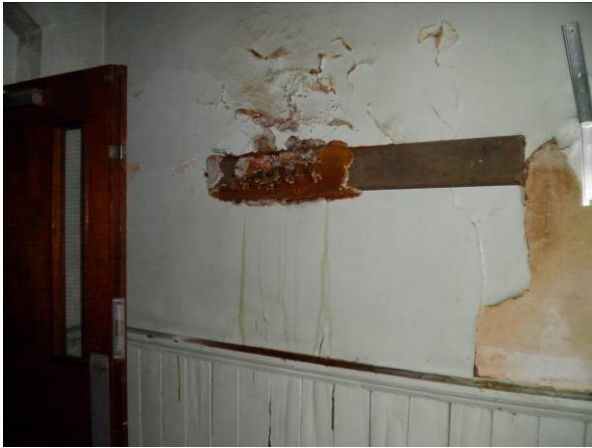
Photo 13 Active dry rot to wall plaster and panelling
