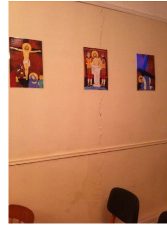
Photo 6 Structural cracking to ground floor
