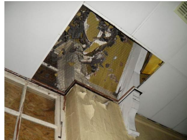
Photo 4 Defective lath and plaster ceiling
