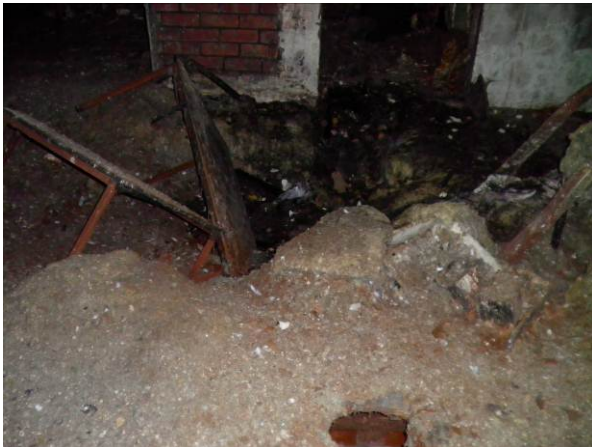
Photo 7 Collapsed floor to central main room
