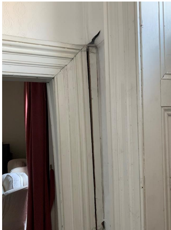
Internal cracking at GF level corresponding with external movement
