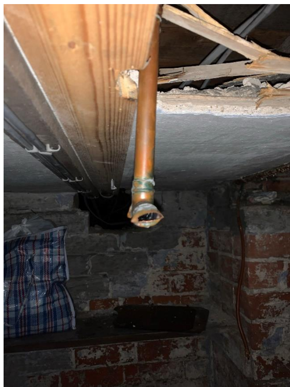
Copper distribution system has been 'stolen'
