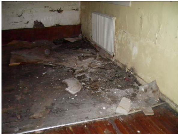
Photo 3 Typical internal view showing damp walls and floors
