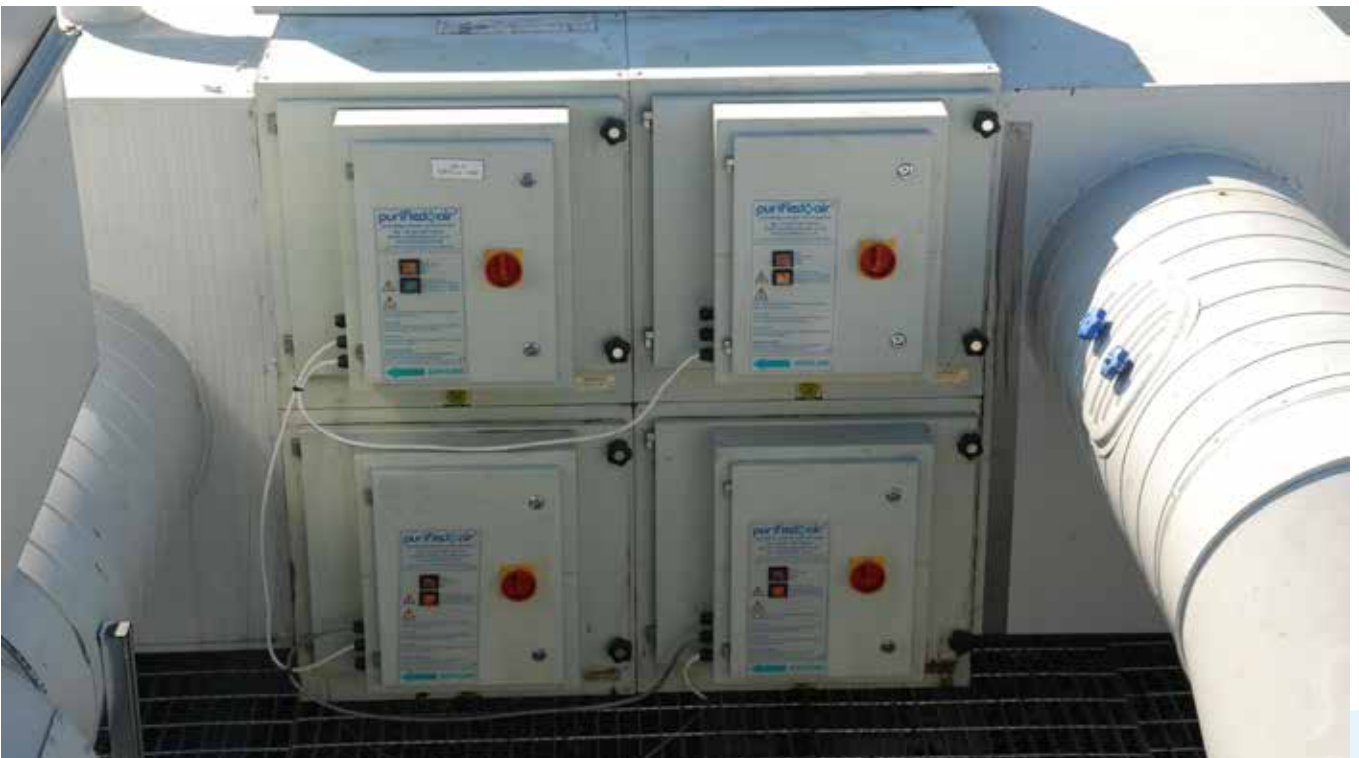
4 ESP Units Stacked in modular formation with a double pass
