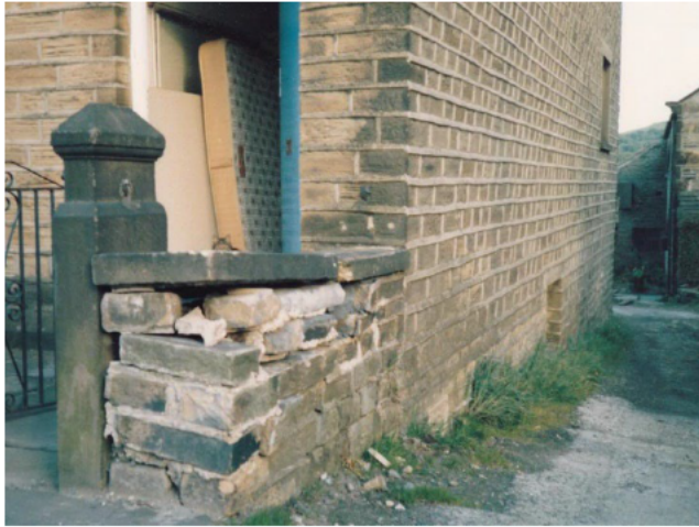
Photo 1: Damage to my front wall from the horse box, about 1986.
