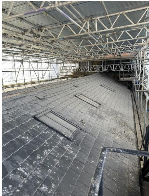
Photo 5. The roof which runs north to south, along the buildings eastern front, showing the scaffolding and cover which prevented a view of the western aspect
