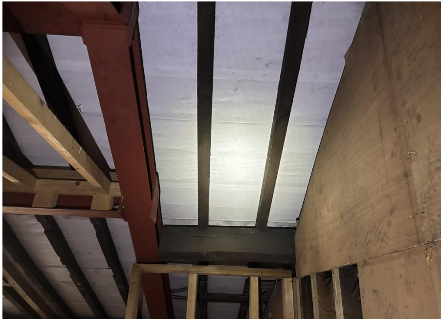
Photo 11. Modern, breathable roof felt, with little to no damage showing lack of suitability for roosting bats
