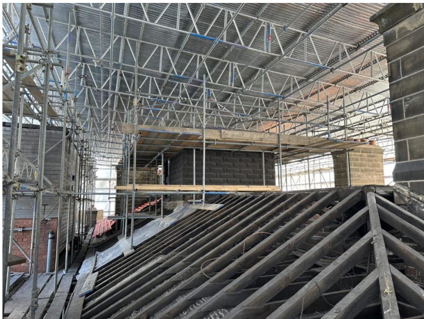
Photo 4. An aspect of the east to west roofline showing further removal works.
