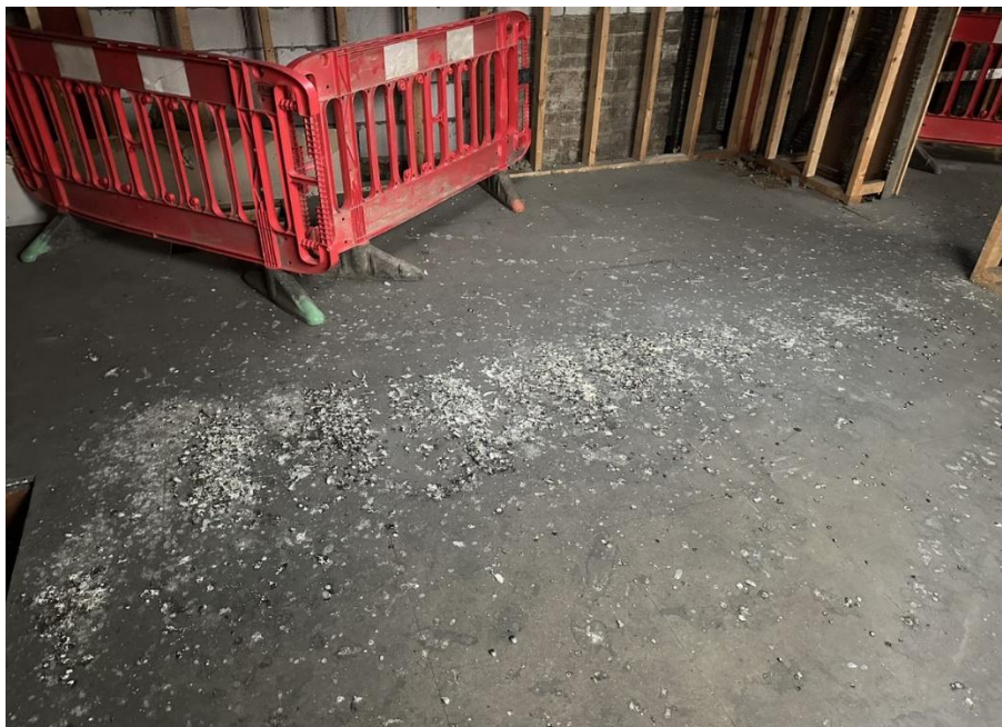
Photo 12. Mounds of pigeon guano in the interior of the building, indicating long-term pigeon presence
