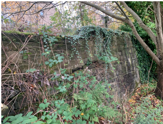
Photograph 7 – Built linear features, poor quality mortared wall featuring cracks/cavities.
