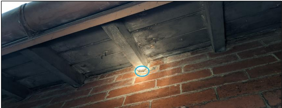
Plate 6. Example of missing mortar beneath ridge tiles
