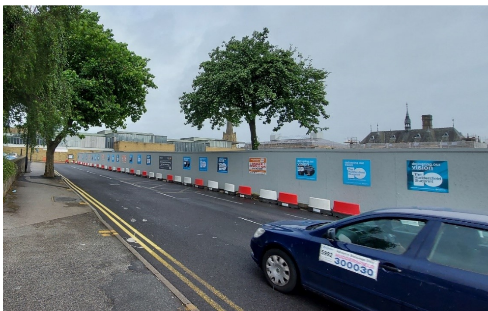
Plate 60: The roof of the Ramsden Building as seen above the fencing across the site of the former car park.
