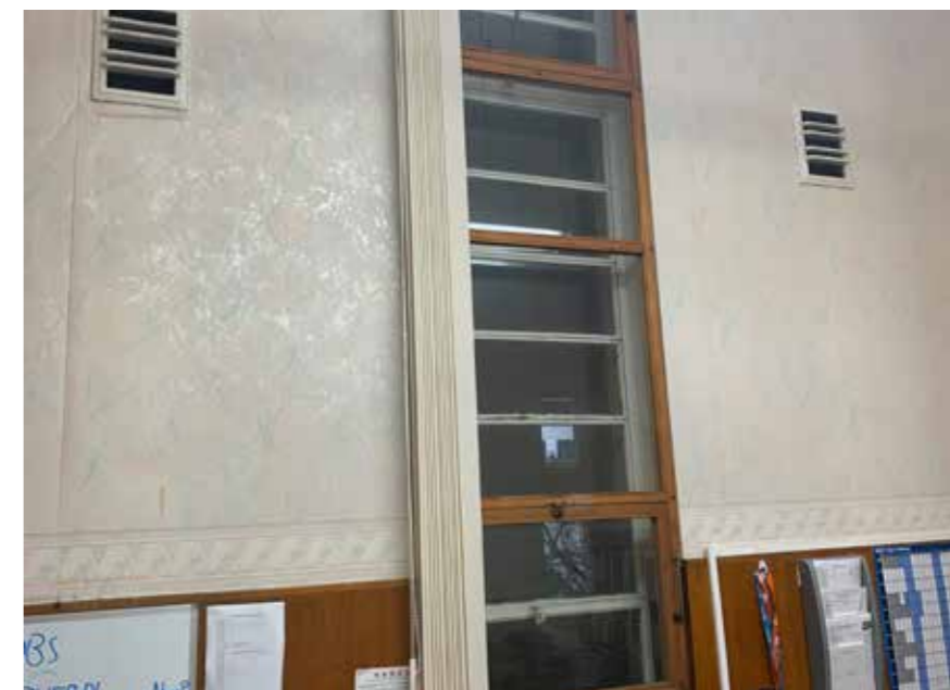
Wall paper (1980s) and secondary glazing (1950s) to the Chief Librarian's Office
