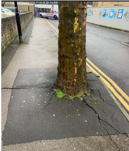
Figure 1: T1 illustrating damage to the pavement.
