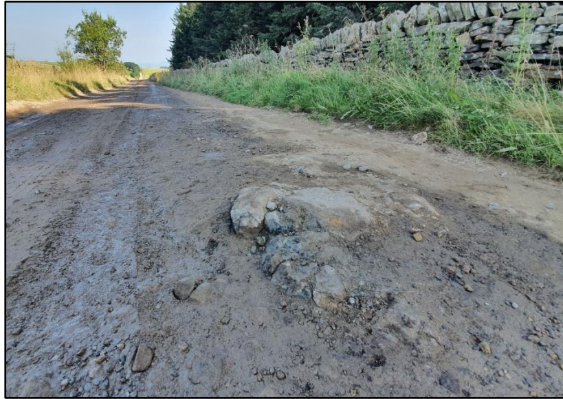
Cartworth Moor Road – Existing uneven surface
