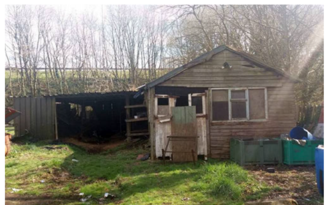
Photo 4: Suitable for a habitable dwelling?
