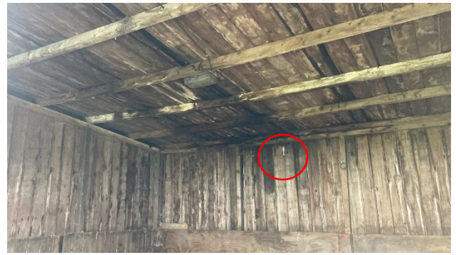
Photo 8: The interior of Building 1. Small cracks in the wood visible.
