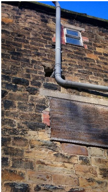
Photo 15-Rear No 4 showing hole
