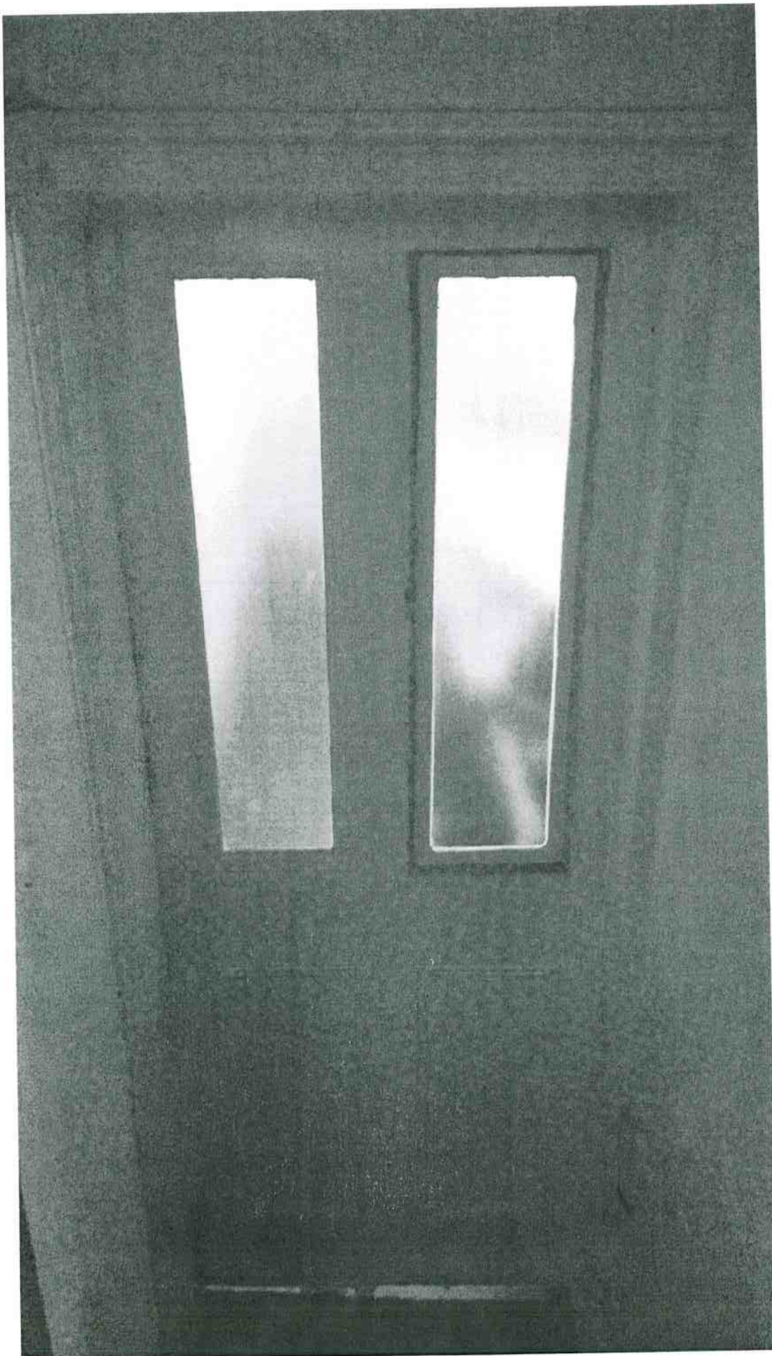
Above shows the door at the bottom of the stairs that requires replacement for fire safety.
