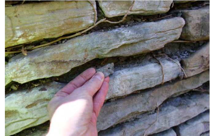
Deeply recessed joints at lower levels, loose pointing
