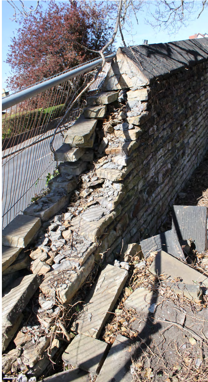
Detail of wall at collapsed end, April 2021
