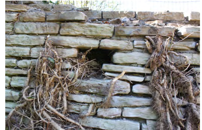
Large voids, open joints and thick roots in the lower sections of the wall facing the motte
