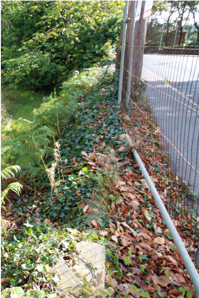
Vegetation cover to lower wall in September 2017
