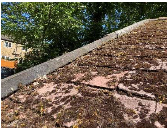
Photograph 7: Small gaps at roof tiles and beneath timber (07.07.2022).
