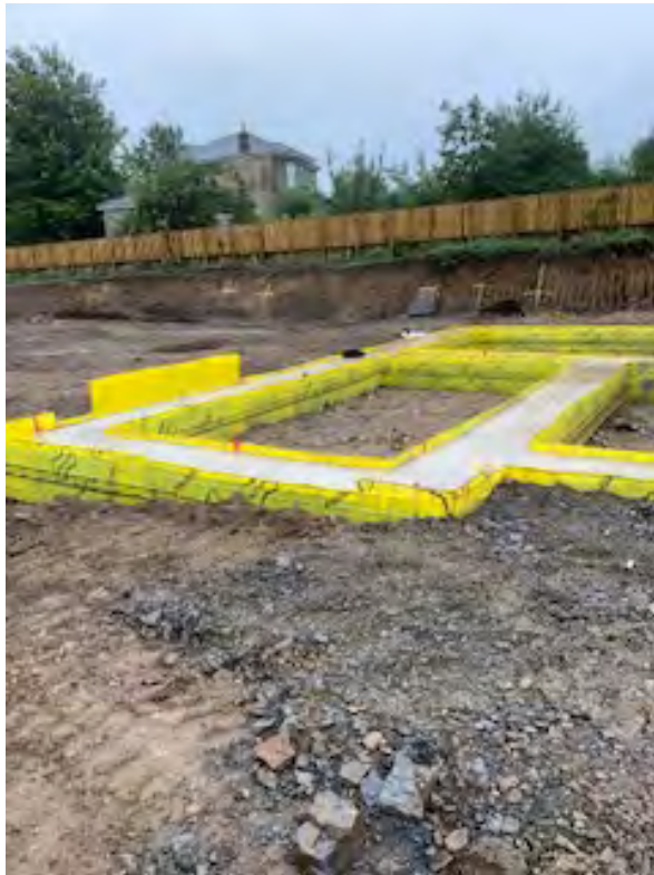
Figure 7 Underfloor Venting Areas
