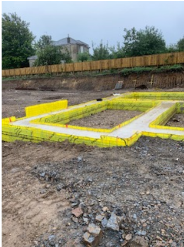
Figure 7 Underfloor Venting Areas
