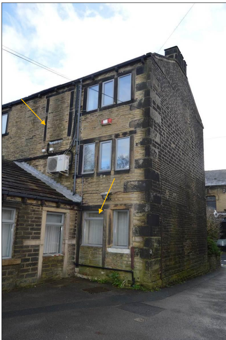
Photograph 14: North wall (facing south) with hoist door and possible cottage doorway (indicated) surrounds in situ .
