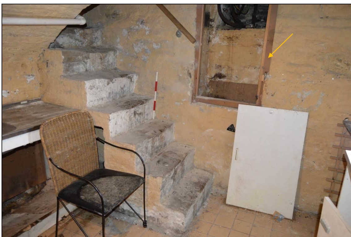
Photograph 16: Stone steps to cellar with former window splay indicated to north elevation (facing north). Scale 0.5m.
