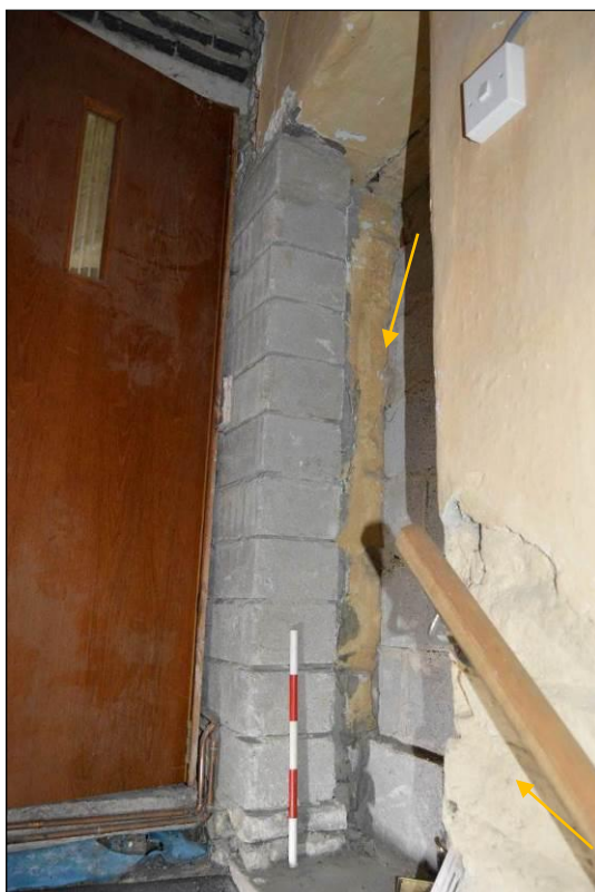
Photograph 20: Former external doorway (stone jamb in situ indicated) in the north elevation now internalised behind the later extension. Scale 0.5m.
