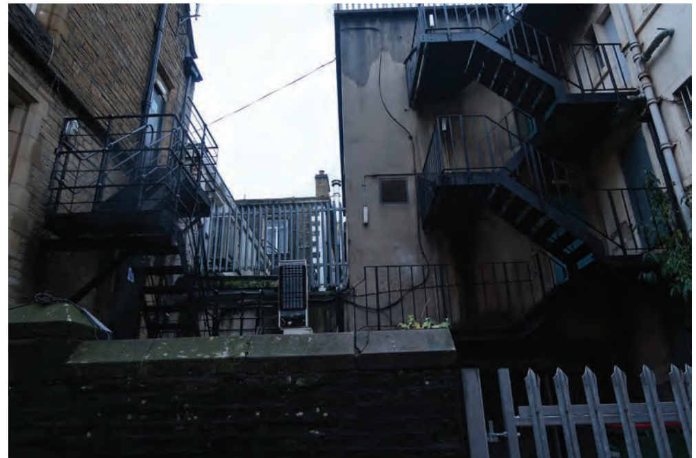
The Albert Yard rear access is currently untidy and functional. The proposal intends to create a new stair tower here in order to access the upper floors from both ends and present a more active and attractive frontage here.
