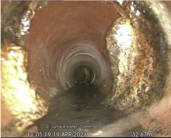
SW1-SW2_32-67m_110519.jpg, 00:07:20, 32.67 m Settled deposits, hard or compacted at joint, 15% cross-sectional area loss
