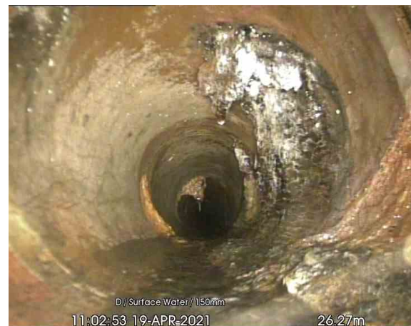
SW1-SW2_26-27m_110253.jpg, 00:05:53, 26.27 m Settled deposits, hard or compacted at joint, 5% cross-sectional area loss
