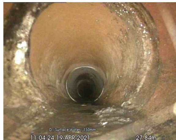
SW1-SW2_27-84m_110424.jpg, 00:06:41, 27.84 m Settled deposits, hard or compacted at joint, 5% cross-sectional area loss
