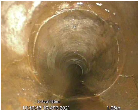
FW 1-FW 2_1-08m_103033.jpg, 00:00:20, 1.08 m Broken pipe at joint from 7 o'clock to 5 o'clock ,
