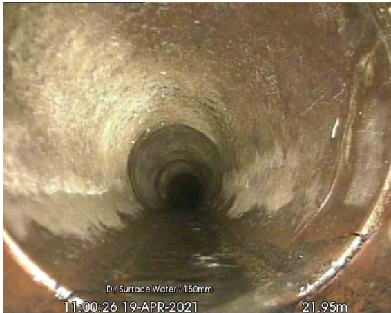
SW1-SW2_21-95m_110026.jpg, 00:04:04, 21.95 m Fracture, circumferential at joint from 2 o'clock to 4 o'clock
