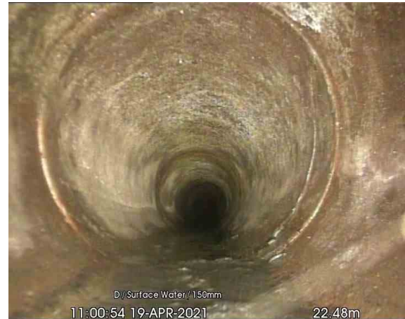
SW1-SW2_22-48m_110054.jpg, 00:04:21, 22.48 m Crack, circumferential at joint from 1 o'clock to 5 o'clock
