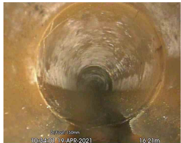
FW 1-FW 2_16-21m_103401.jpg, 00:02:38, 16.21 m Crack, circumferential at joint from 8 o'clock to 11 o'clock
