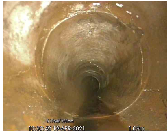
FW 1-FW 2_1-09m_103042.jpg, 00:00:23, 1.09 m Fracture, longitudinal at 4 o'clock
