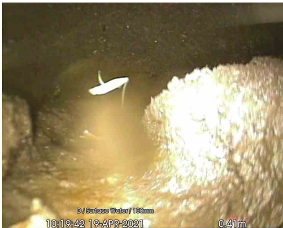
GY2_0-41m_101942.jpg, 00:00:09, 0.41 m Settled deposits, fine, 50% cross-sectional area loss
