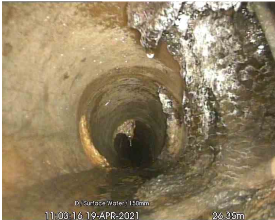
SW1-SW2_26-35m_110316.jpg, 00:06:08, 26.35 m Settled deposits, hard or compacted, 20% cross-sectional area loss
