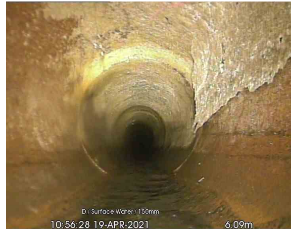
SW1-SW2_6-09m_105628.jpg, 00:01:16, 6.09 m Settled deposits, hard or compacted, 5% cross-sectional area loss
