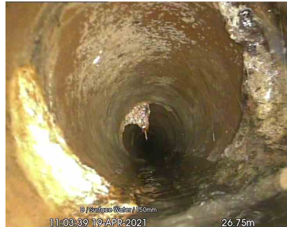
SW1-SW2_26-75m_110339.jpg, 00:06:18, 26.75 m Settled deposits, hard or compacted at joint, 10% cross-sectional area loss
