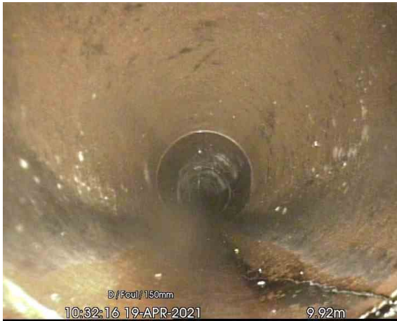
FW 1-FW 2_9-92m_103216.jpg, 00:01:24, 9.92 m Fracture, longitudinal at joint at 5 o'clock
