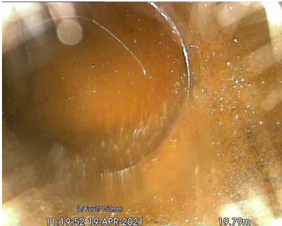
FW 1- A_19-79m_111952.jpg, 00:01:06, 19.79 m Crack, circumferential at joint from 9 o'clock to 2 o'clock
