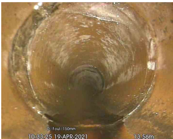
FW 1-FW 2_13-56m_103325.jpg, 00:02:11, 13.56 m Crack, circumferential at joint from 6 o'clock to 11 o'clock
