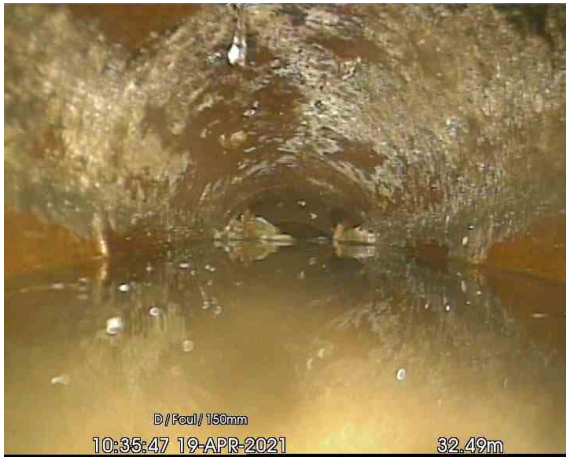
FW 1-FW 2_32-49m_103547.jpg, 00:04:11, 32.49 m Water level, 80% of the vertical dimension, BLOCKED
