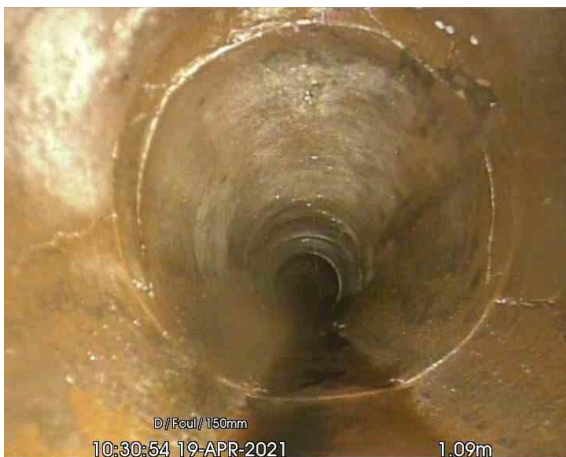
FW 1-FW 2_1-09m_103054.jpg, 00:00:26, 1.09 m Crack, longitudinal at 8 o'clock
