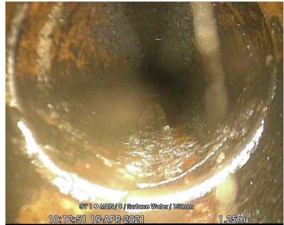
KNOWLE GROVE_1-25m_101251.jpg, 00:00:29, 1.25 m Fracture, circumferential at joint from 4 o'clock to 6 o'clock
