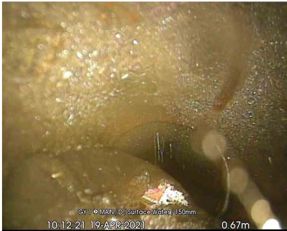
KNOWLE GROVE_0-67m_101221.jpg, 00:00:12, 0.67 m Settled deposits, fine, 70% cross-sectional area loss
