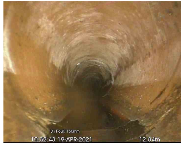
FW 1-FW 2_12-84m_103243.jpg, 00:01:41, 12.84 m Crack, circumferential at joint from 4 o'clock to 8 o'clock
