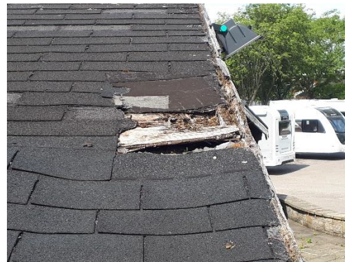
Image 15: Close up of potential roost feature (B1)
