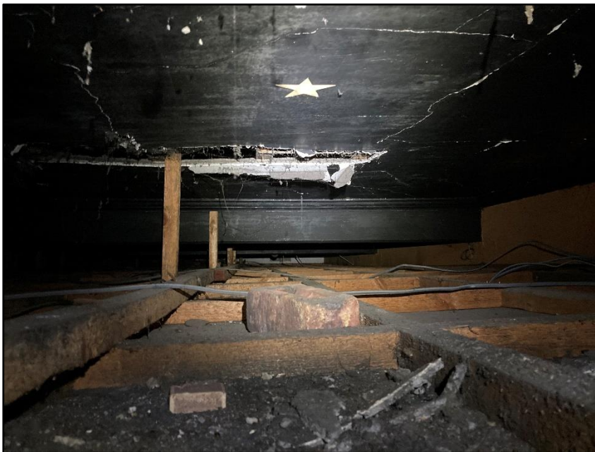
Photograph 25 showing the small void between the underside of the flat roof and the suspended ceiling
