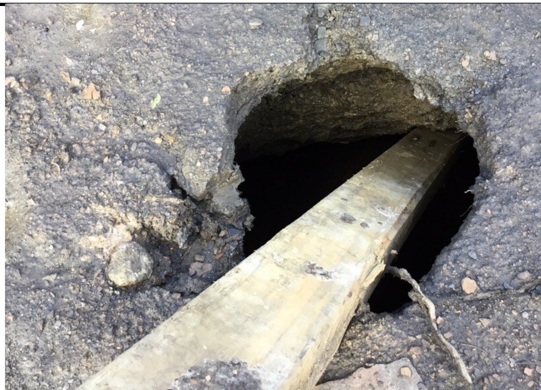
Photo 2: Hole had opened in the centre of site prior to site investigation.
