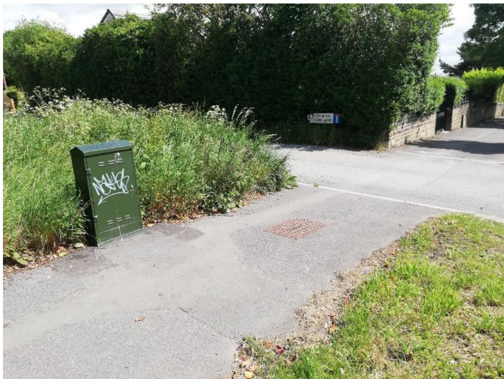
Photograph 1: Utility Cabinet and underground services chamber at the end of Shepherds Thorn Lane
