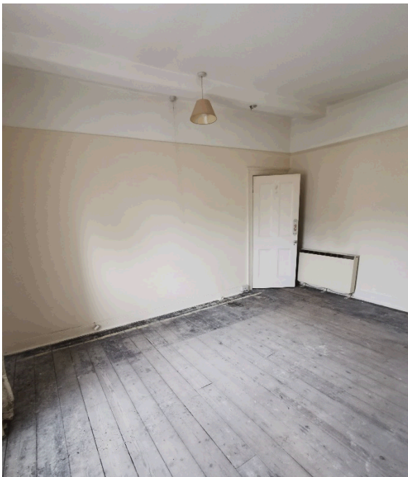
Photograph 14 - Bedroom 3 showing no ceiling cornice/coving details
