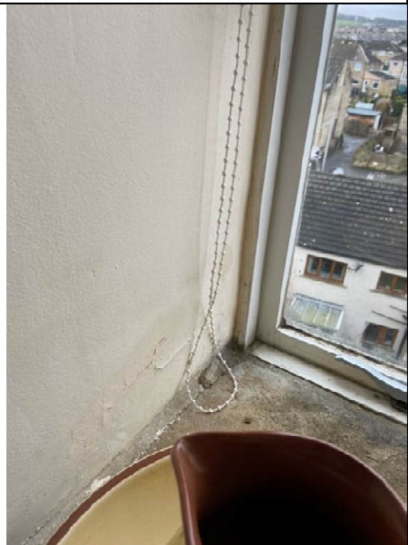
First floor (second floor when looking at back elevation) Internal showing damage to wall and stone due to leaks
