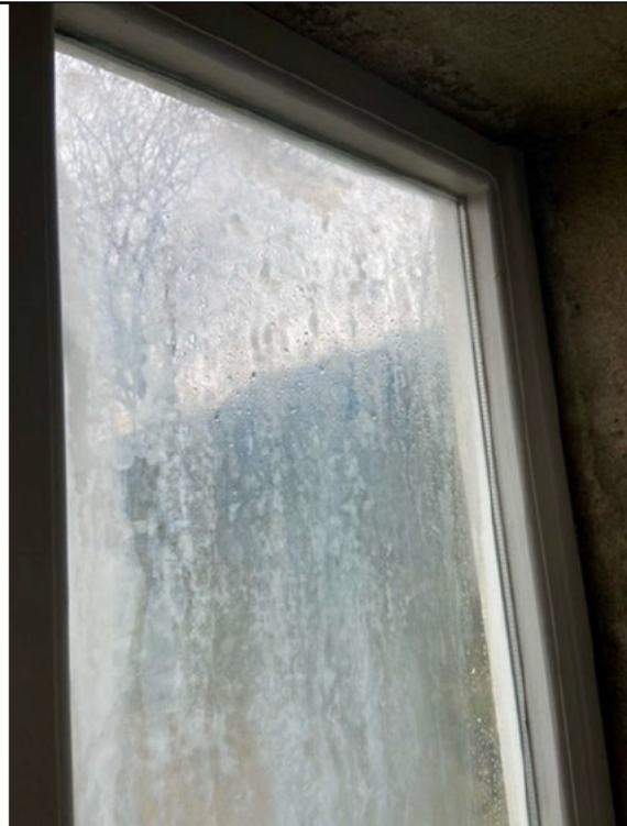
Internal lounge window showing blown glass
