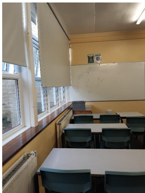
Fig 3: Existing Classroom, external glazing
