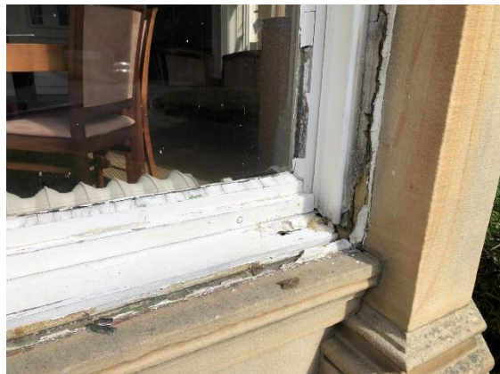
Photo 15 – Current condition of timber windows
