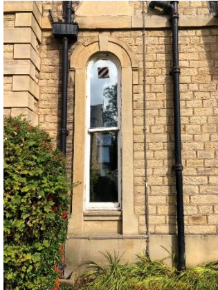
Photo 16 – Current condition of timber windows
