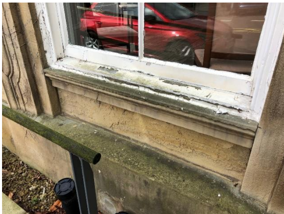
Photo 14 – Current condition of timber windows
